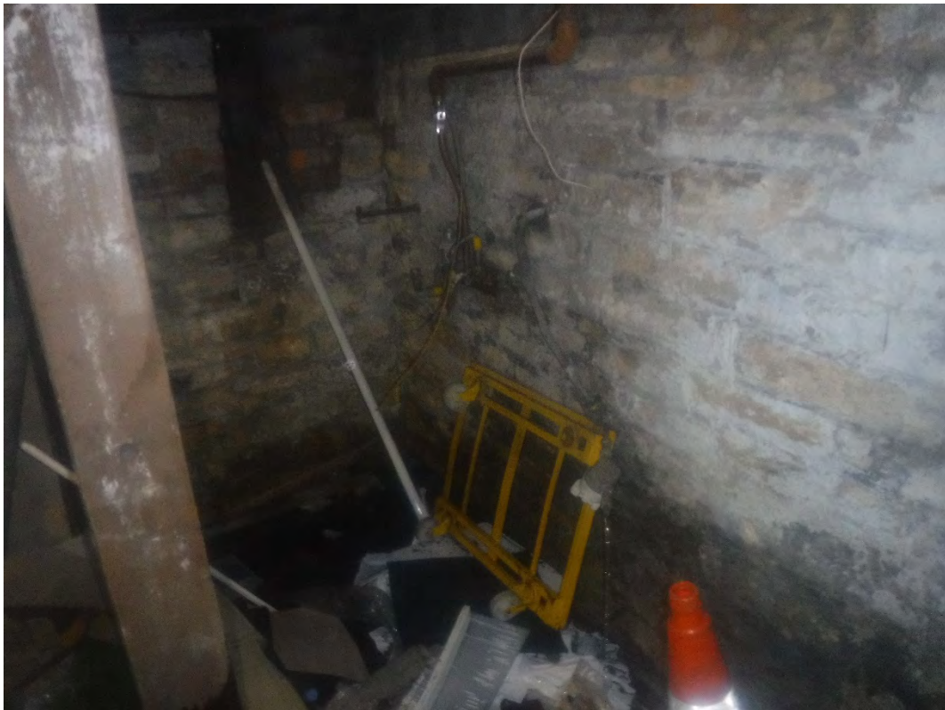
Photograph No.5: Running tap causing a leak on southern edge of basement level
