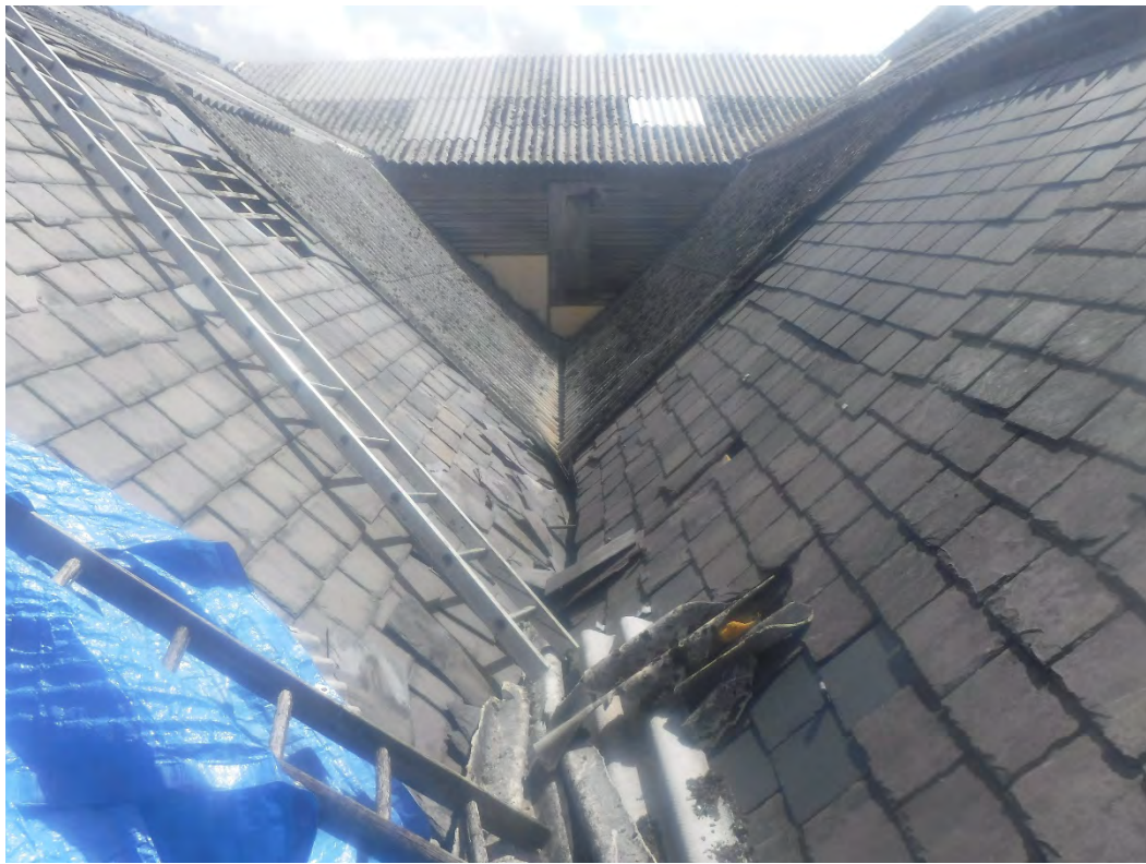
Photograph No.11: Roof as seen from top floor showing mix of slate and asbestos tiles
