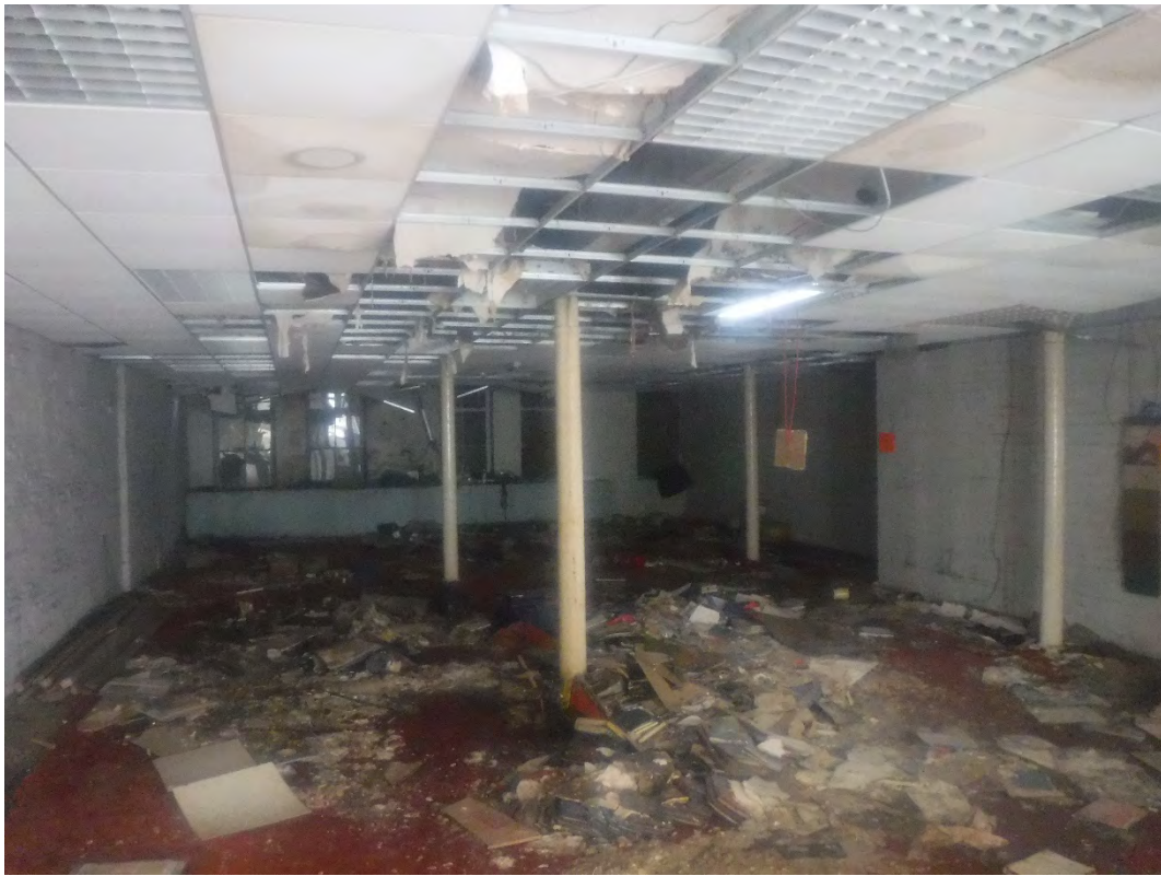
Photograph No.7: First floor, carpet soaked with water
