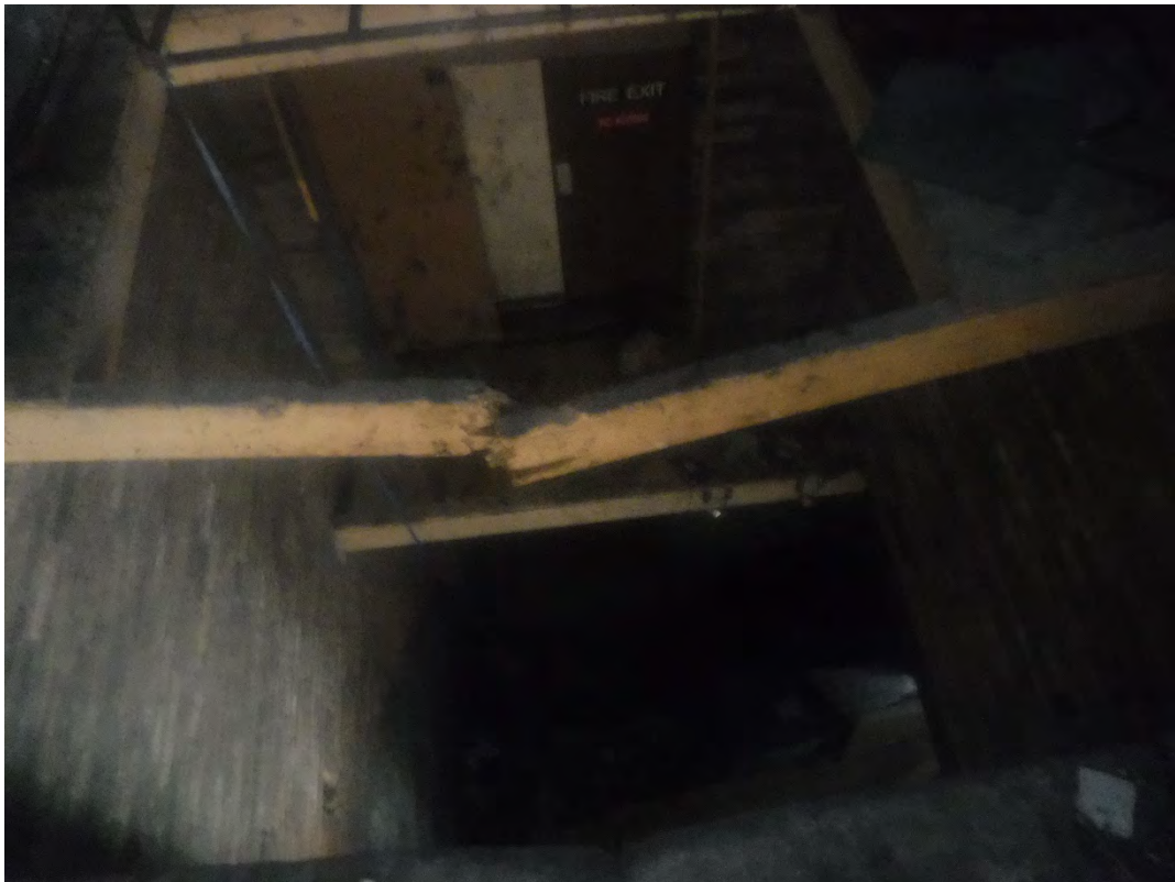
Photograph No.14: Lift shaft in south east part of site extending from ground floor to roof level
