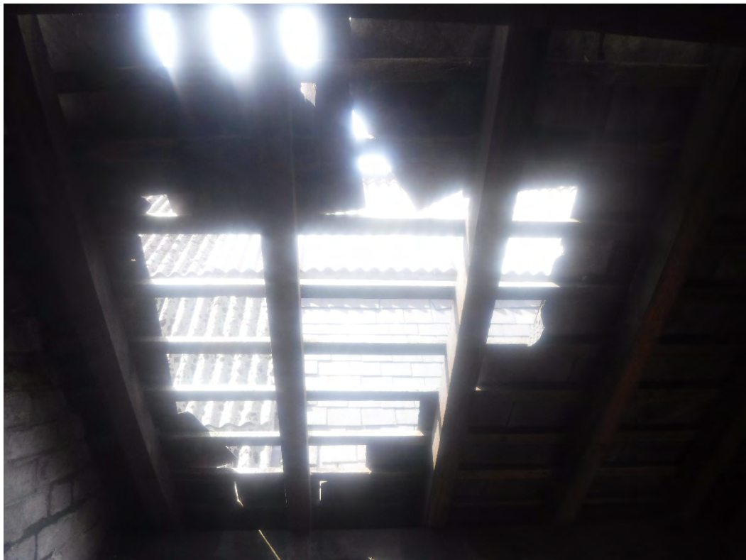
Photograph No.12: Roof level showing holes in structure
