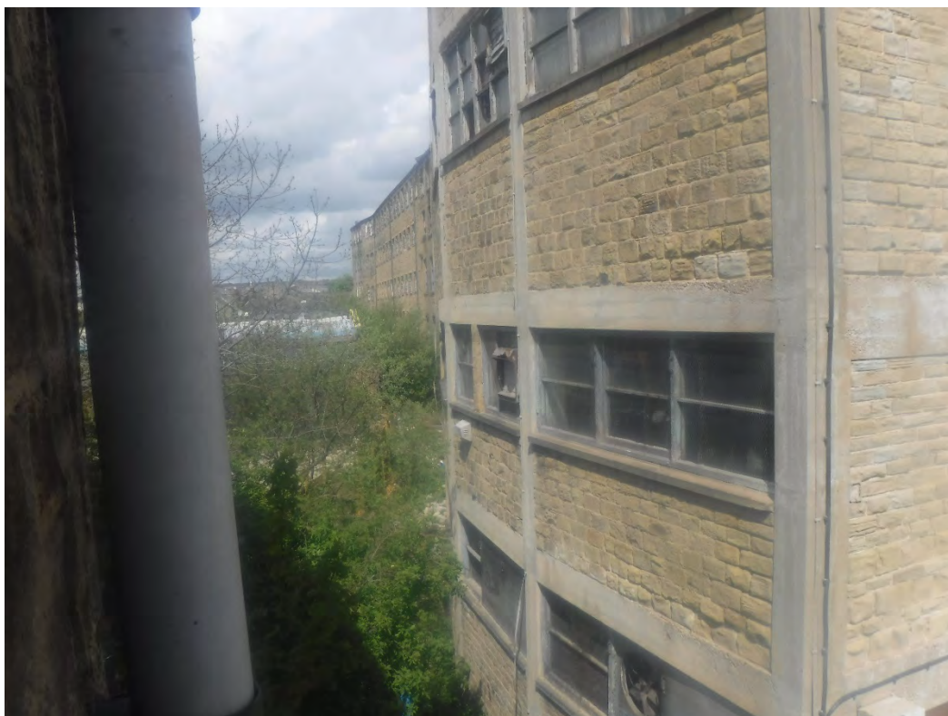
Photograph No.10: Mill buildings to the north west from second floor window
