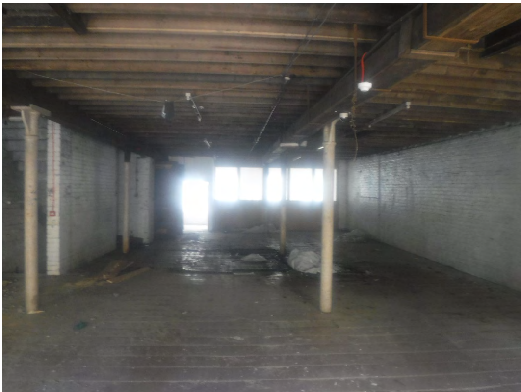
Photograph No.8: Second floor, damp section in centre
