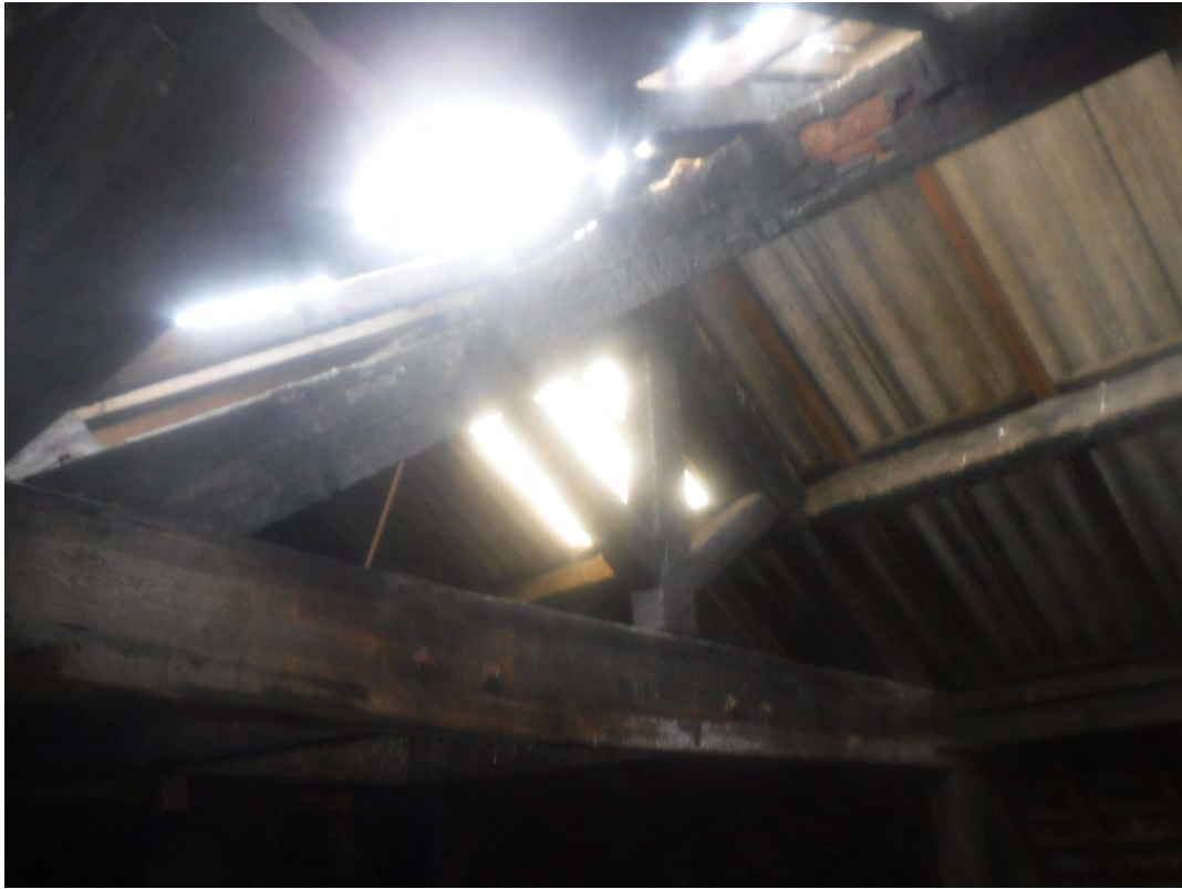
Photograph No.13: Another view of roof with holes in structure
