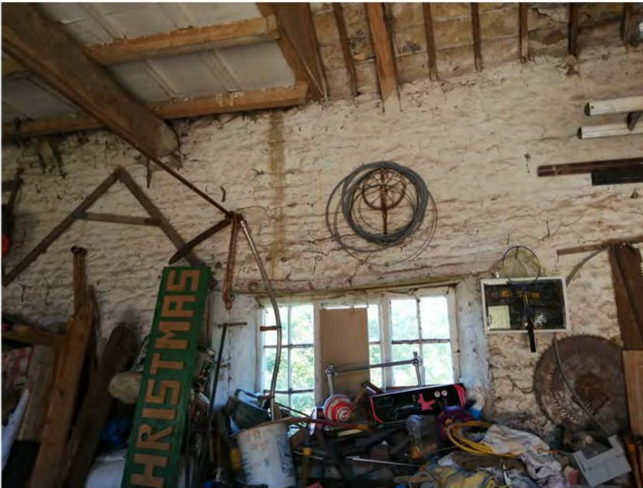
Plate 12 Looking East at Deflecting Lintel in Workshop Eastern Elevation Opening
