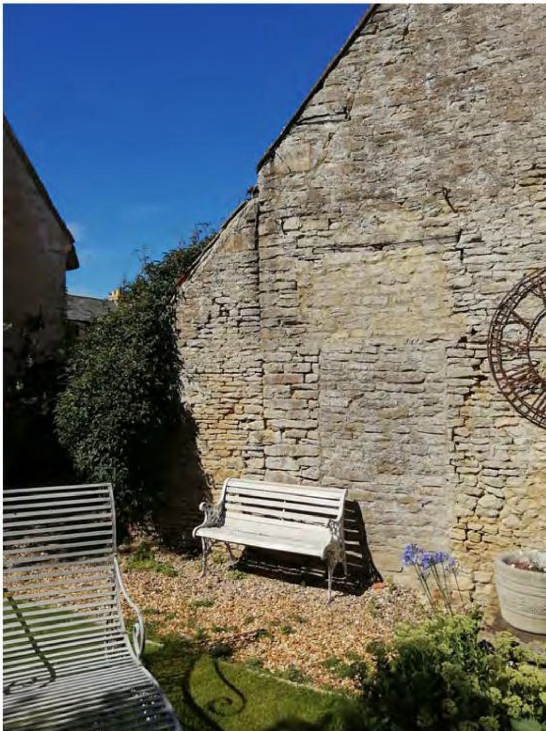
Plate 6 Looking North at Cracking to Infill Panel in Southern Gable Elevation
