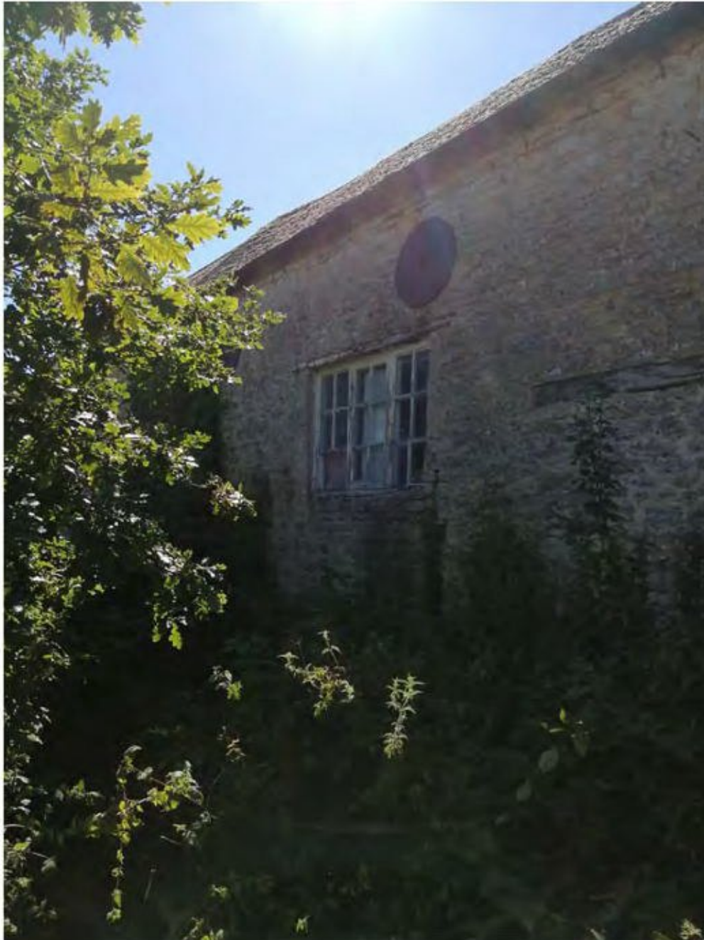
Plate 9 Looking South West Along Eastern Elevation at Poor Timberwork to Windows and Supporting Lintel Above
