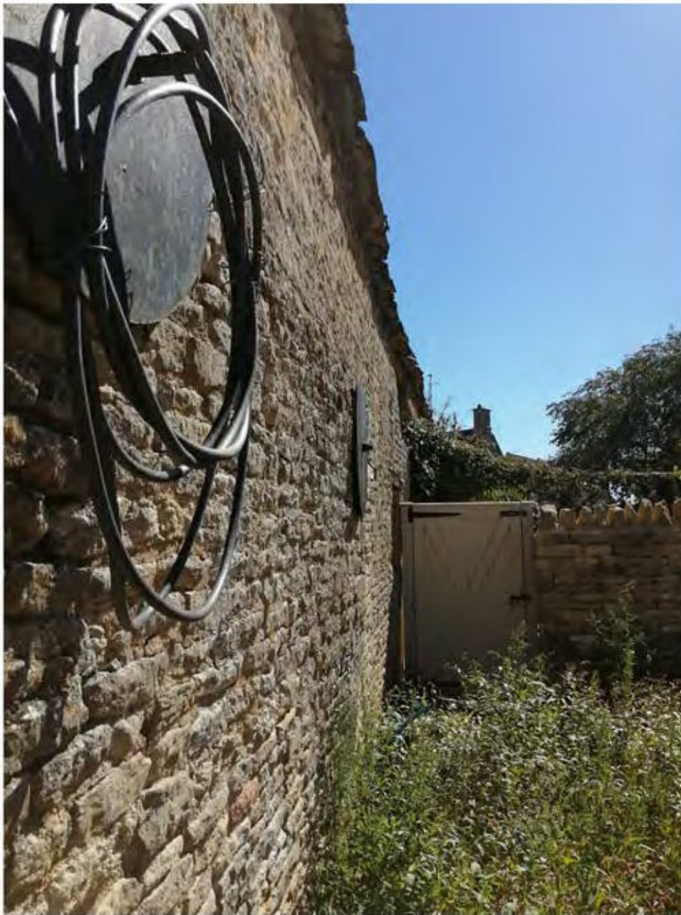
Plate 3 Looking South West Along Flank Wall at Bellying Stonework at Wallplate Level
