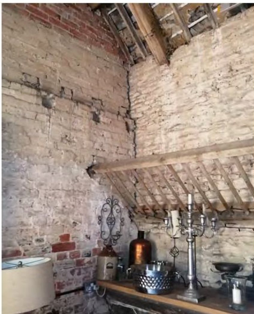
Plate 10 Looking East at Vertical Cracks Between Eastern Flank Wall & Cross Wall
