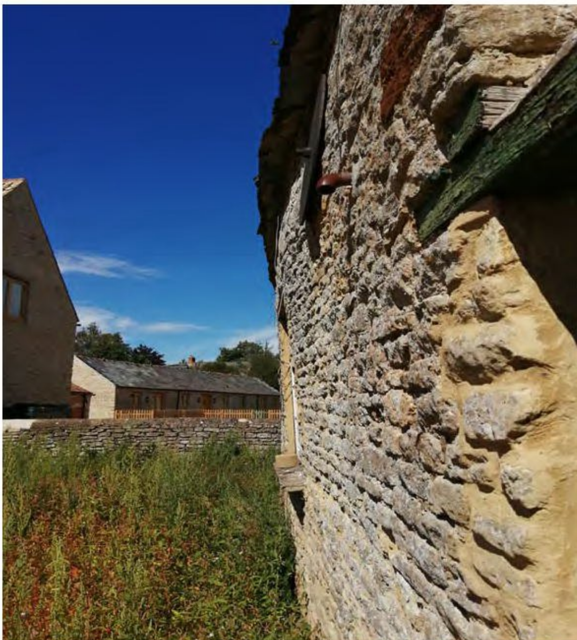
Similarly, further along to the north of this flank wall, the stonework is bellying outwards (Plate 4). Note the bulge is worse over the window opening to the workshop.
