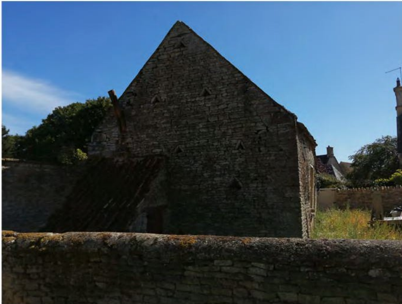
Plate 7 Looking South at Cracking in North East Gable End
