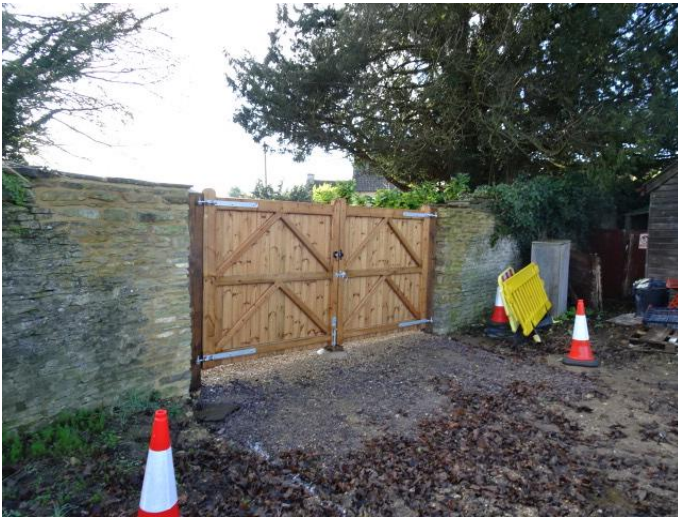
New gates part of works to provide access to sewage treatment plant
