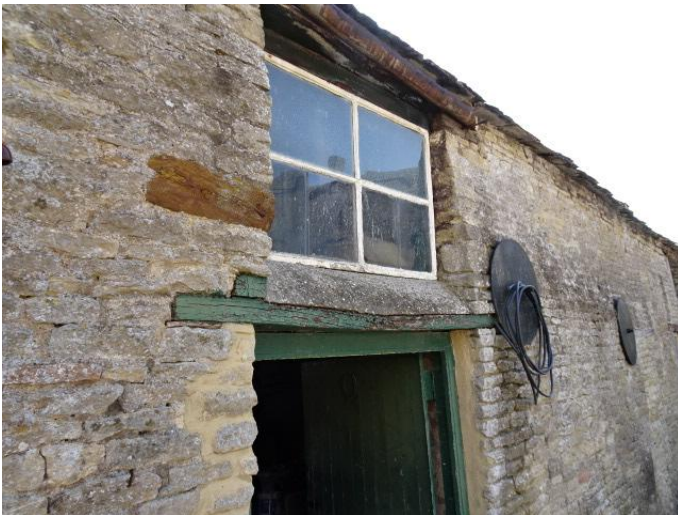
Bulging wall (northwest corner)
