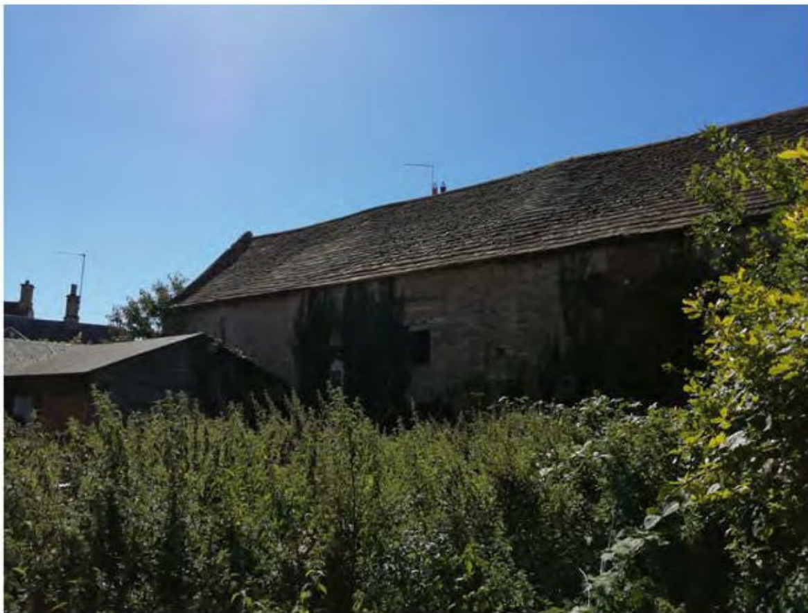
Plate 8 Looking West at Undergrowth Abutting and Growing Up East Facing Flank Wall
