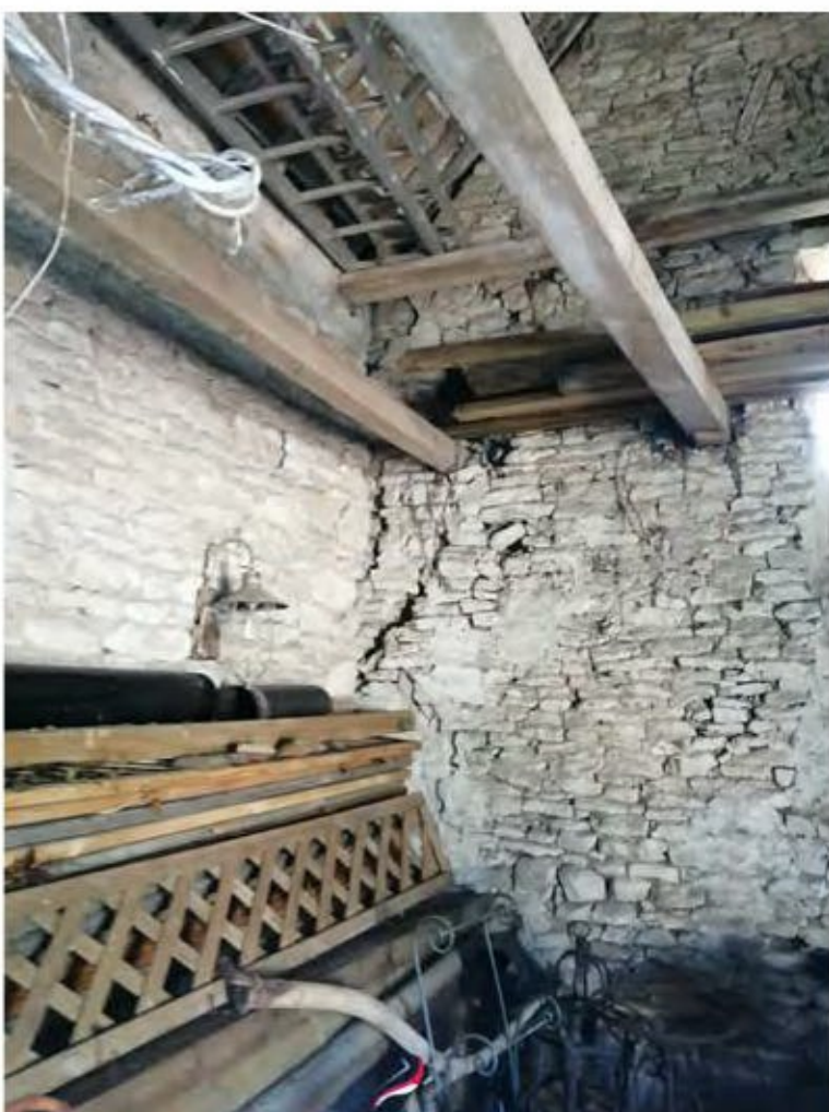
Plate 12 Looking South at Internal Gable Wall Where Cracking Exists Where Intersecting with Eastern Flank Wall
