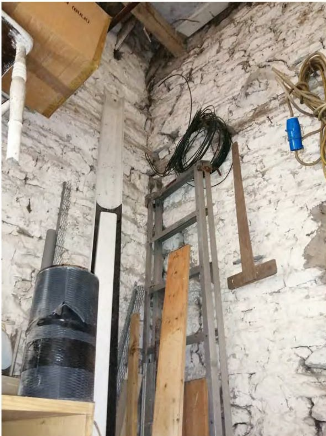
Plate 15 Looking North West at Vertical & Diagonal Cracking to Stonework
