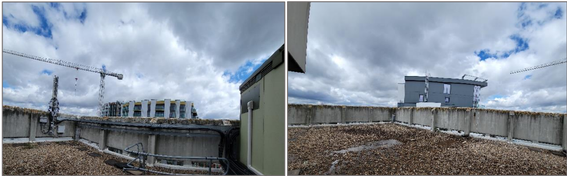
Images from the 13 th floor roof of Riverside House. Neighbouring buildings visible but no direct view of any rooftop plant or any audible plant.
