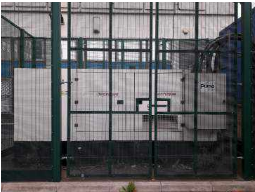
PHOTO 8: The fuel generator as taken during a previous visit to site in September 2018.
