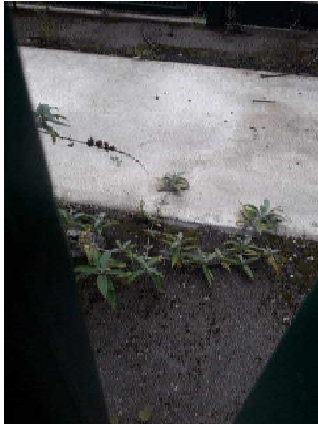
PHOTO 7: Concrete slab below the former fuel generator. Slightly darker staining on the concrete was observed towards the right hand side of this photograph.
