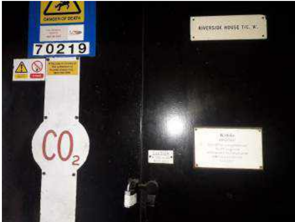
PHOTO 3: One of the electricity substations.
