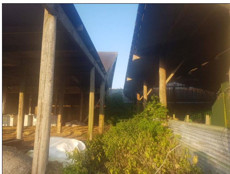
Figure 6. Encroaching vegetation along southern edge of building.
