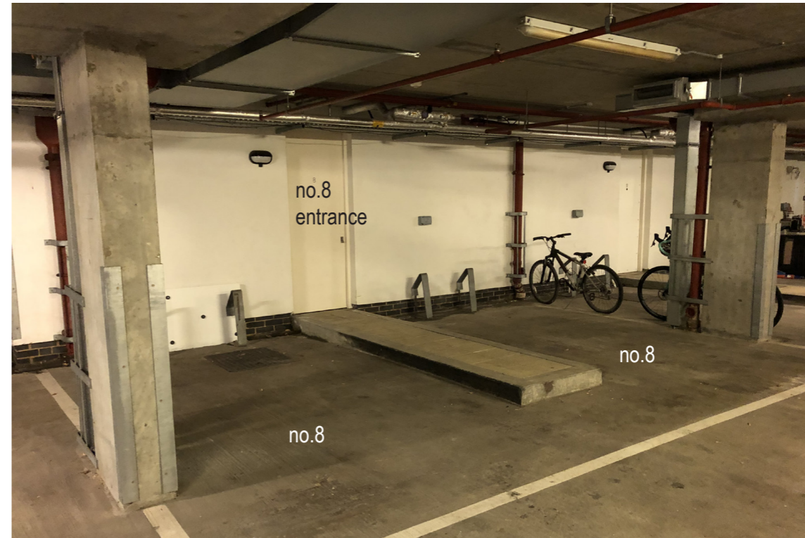
Existing side to side parking to no.8 (note the entire footprint of no.8 continues to basement level)
