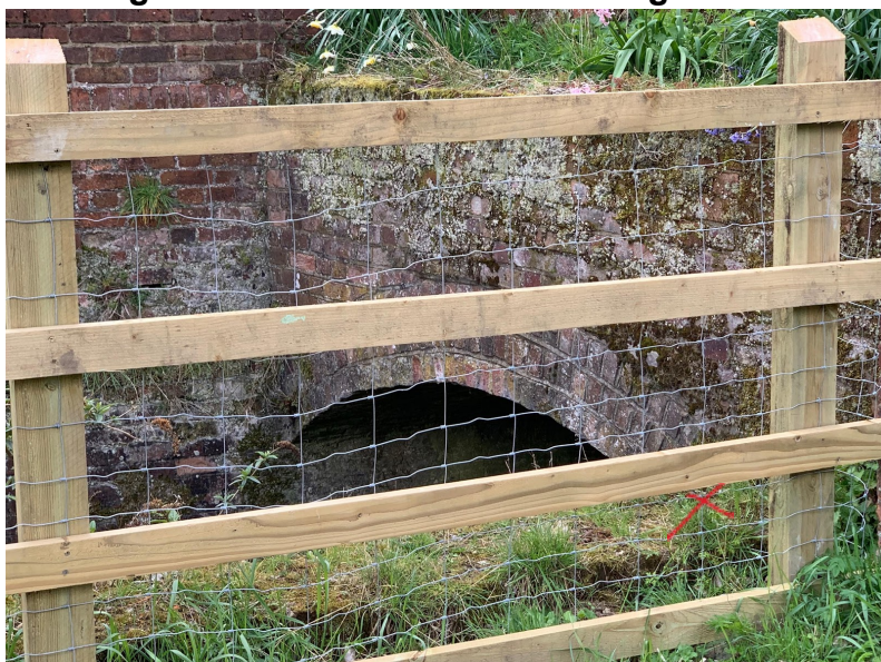
Photo 16. View of bridge facing south west of the house. Red cross is where we would like to add light.
