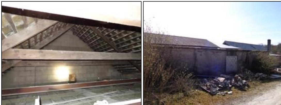
Figures 2 & 3. Interior view of [pitched slate] roof void; building viewed from the north
