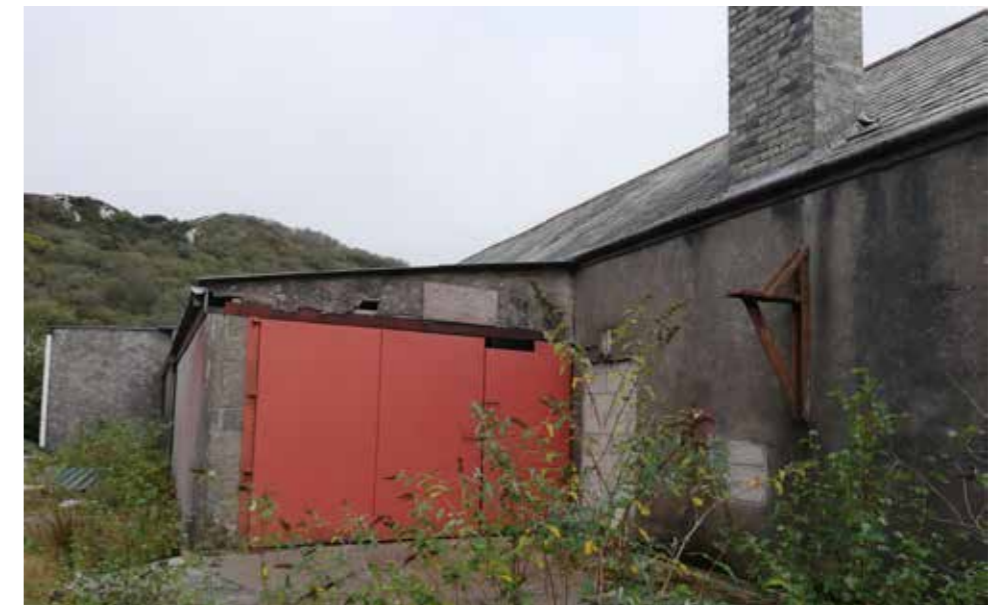
Disjointed rear elevation indicating poor state of existing building
