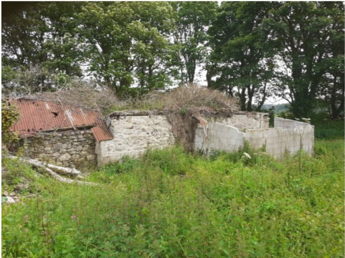
Figure 4: Photo showing the North West elevation of the existing building. The proposed dwelling sits on the same footprint as the existing building, with the existing stonework structure retained.
