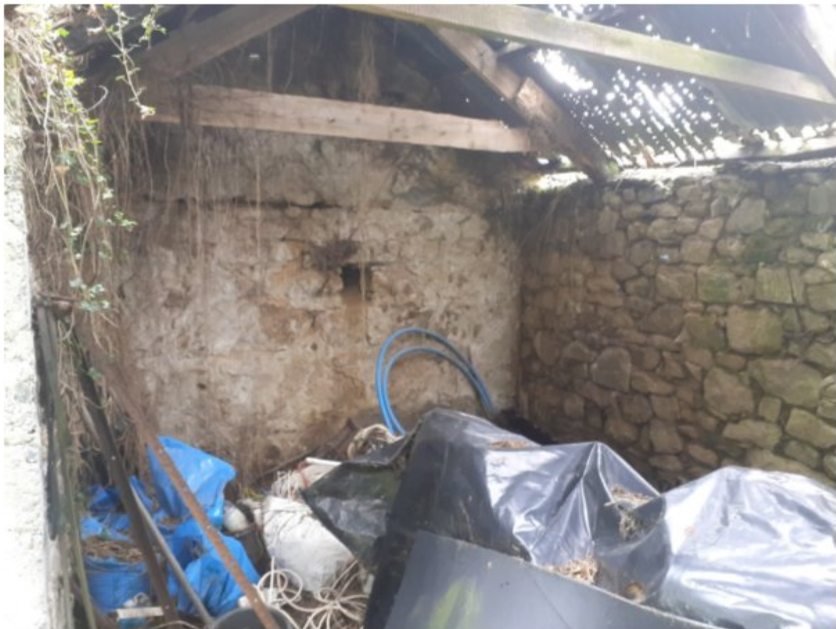
Figure 5: Photo of the inside of the existing building, showing the existing stonework walls which are generally in good condition and will be retained within the development.
