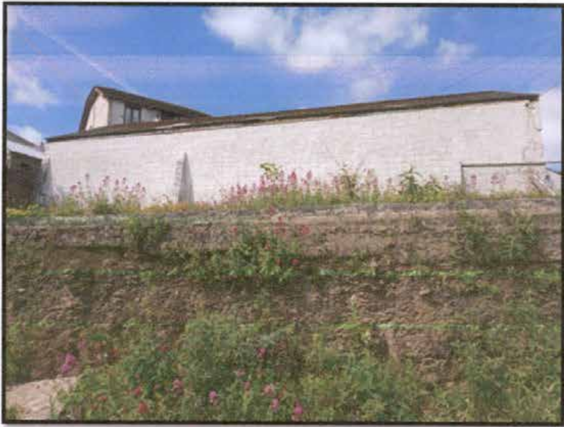
Photograph 5 – View of exposed rock and concrete slab covering Upper Level, looking west.
