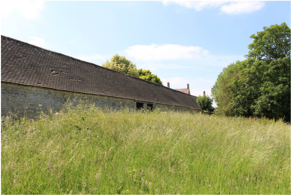
Image EDP 4: View of the east elevation of the former shelter shed looking northwest showing the relatively blank wall, with only the two former doors.
