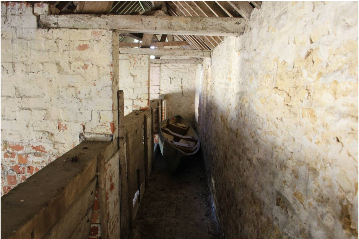
Image EDP 15: View of the interior of the later section of the piggery, looking south.
