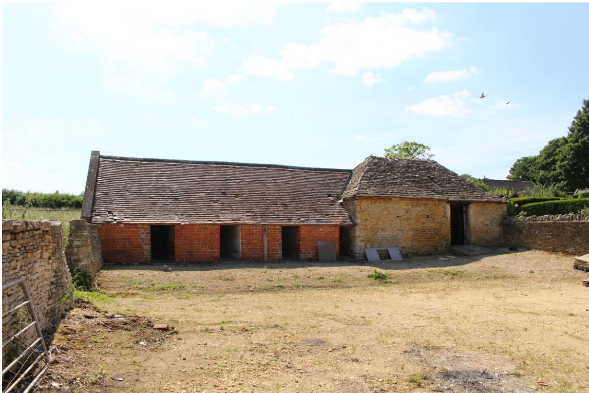
Image EDP 13: View of the piggyery, with the early section to right and the later section to left, looking west.
