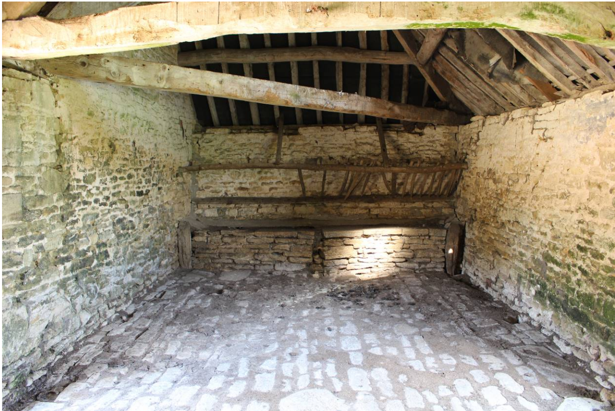
Image EDP 12: View of the southern wing, showing the dilapidated hayrack, the stone bench and cobbled floor, looking east.
