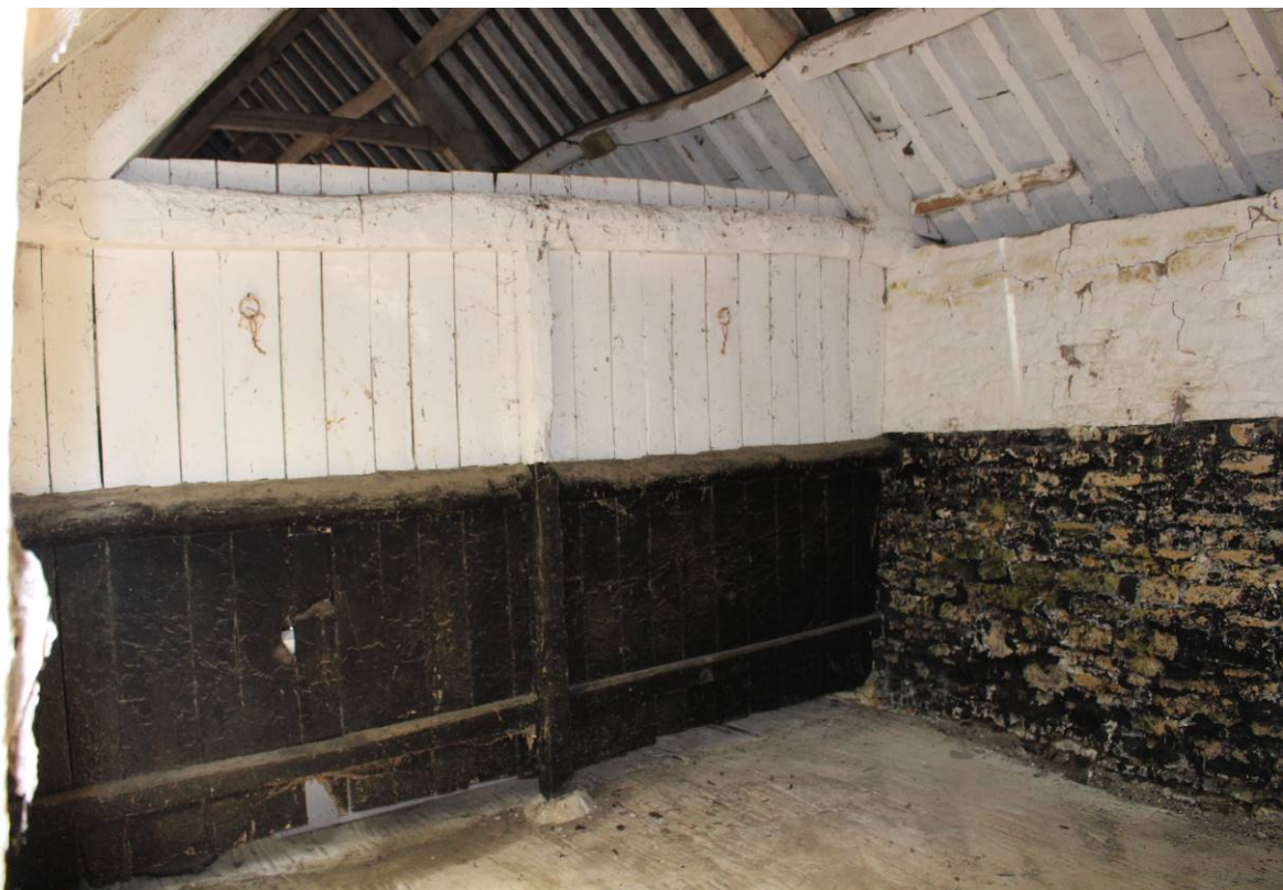
Image EDP 8: View of one of the interior partitions, showing planks attached to framing.
