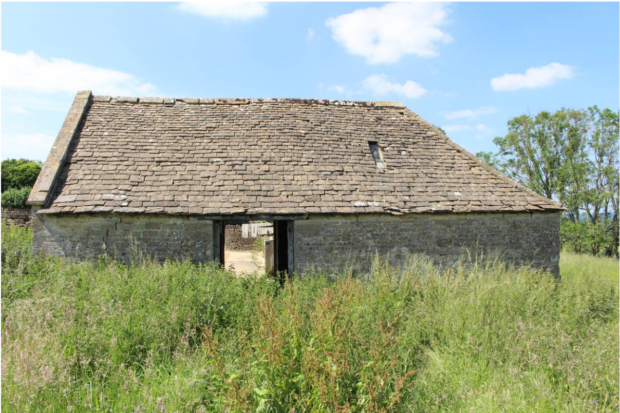
Image EDP 7: View of the southern elevation of the former shelter shed, looking north.
