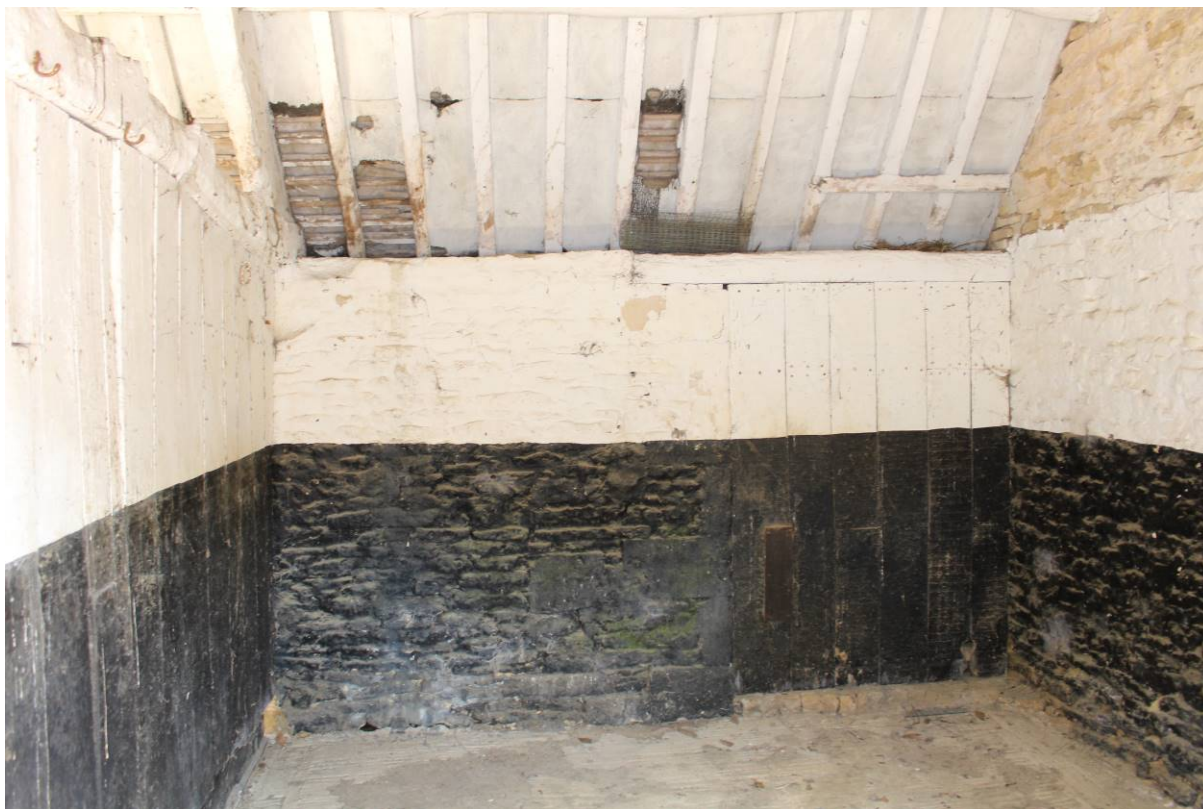
Image EDP 6: View of the interior of a stall, noting the nailed planking on the inside of the former door, looking east.
