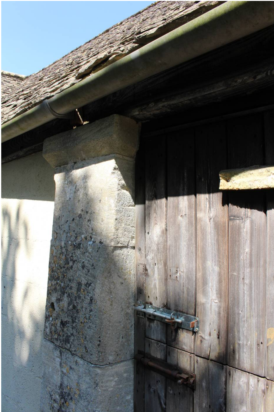
Image EDP 3: View of the detail of a column, showing how the stable door has been cut into the head.
