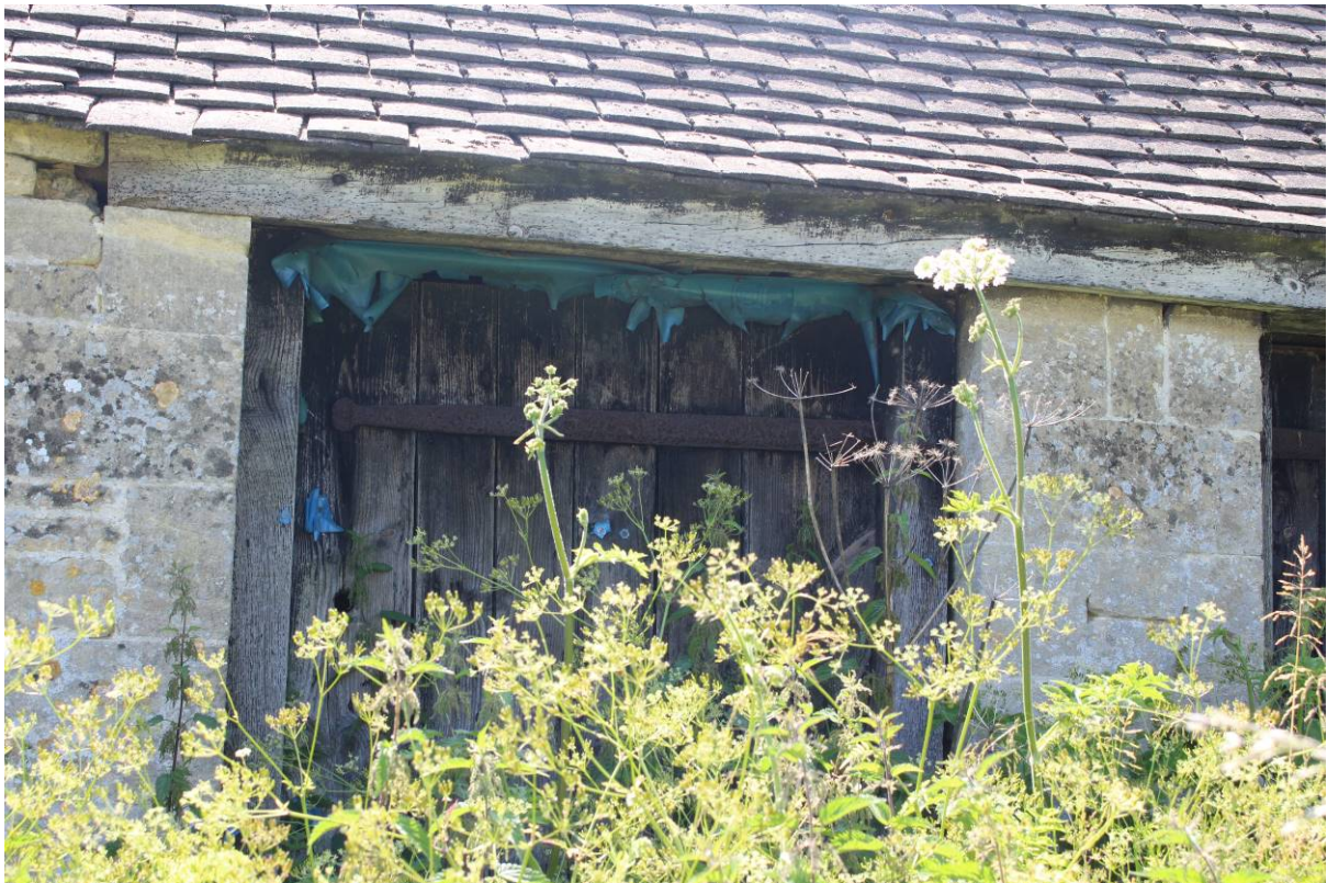
Image EDP 5: View of one of the doors, sealed shut from the inside, most likely of 19 th century date.
