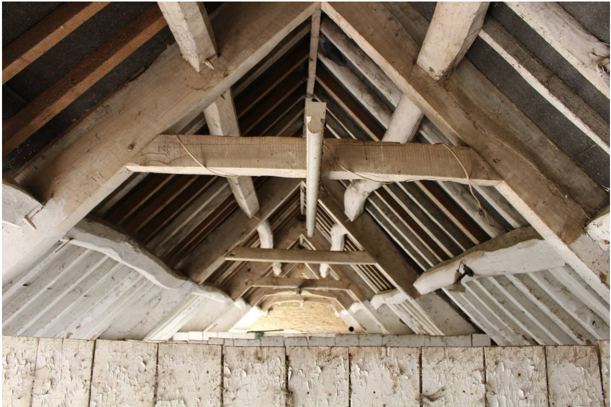
Image EDP 10: View of the roof structure, looking north, note replacement rafters to left.
