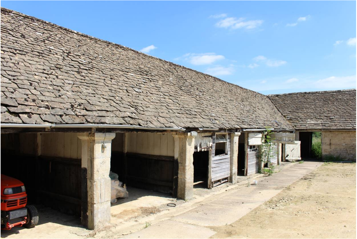
Image EDP 2: View of the former southern end of the former shelter shed, looking south-east.
