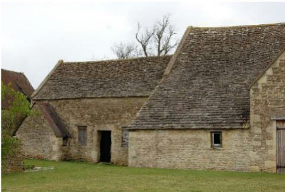
Photograph 5. The north-west section of the south-west elevation of Barn 1. Photograph shows the extension and north-western lean-to (main swarming site)
