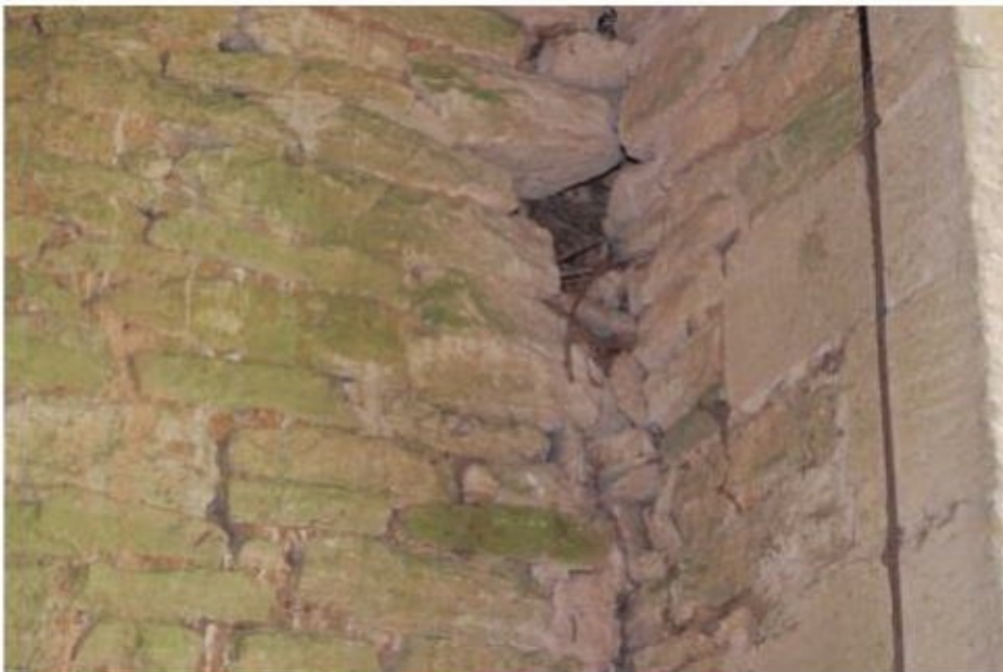
Figure 22. Photograph showing a jackdaw nest within a crevice in Barn 1. South-eastern room of main barn.
