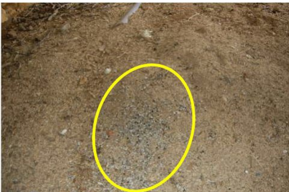
Figure 24. Photograph showing concentration of pigeon droppings. South-eastern room of main barn.
