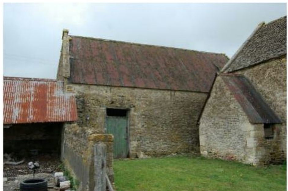
Photograph 12. The south-east elevation of Barn 2-main barn, with a section of Barn 1 viewed to the right of the photograph.
