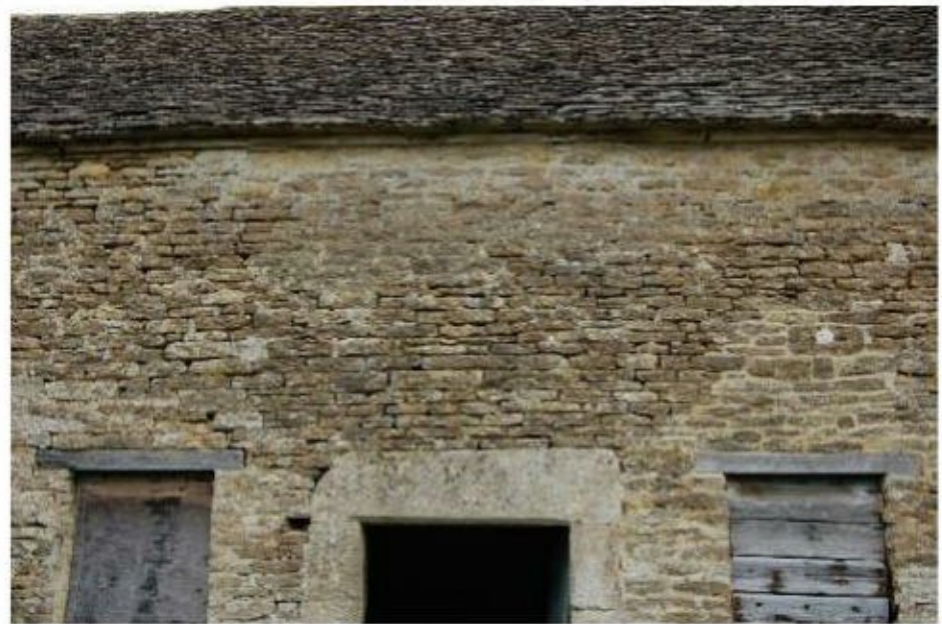
Photograph 10. Photograph showing external crevices between the stonework.
