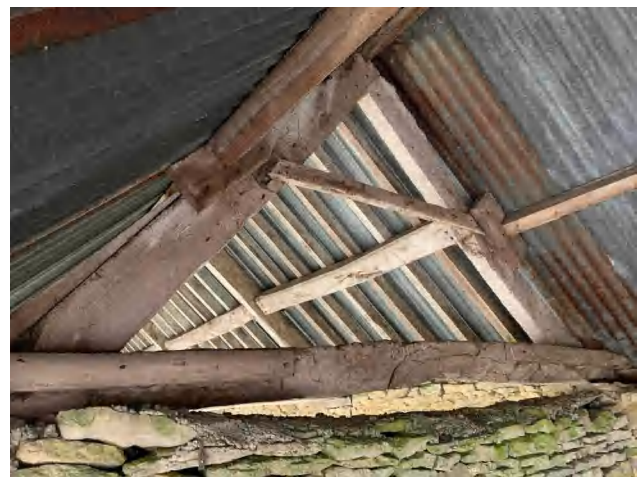
3.58 The roof of Building D, looking south from the central part into the southern three bays (DIA).
