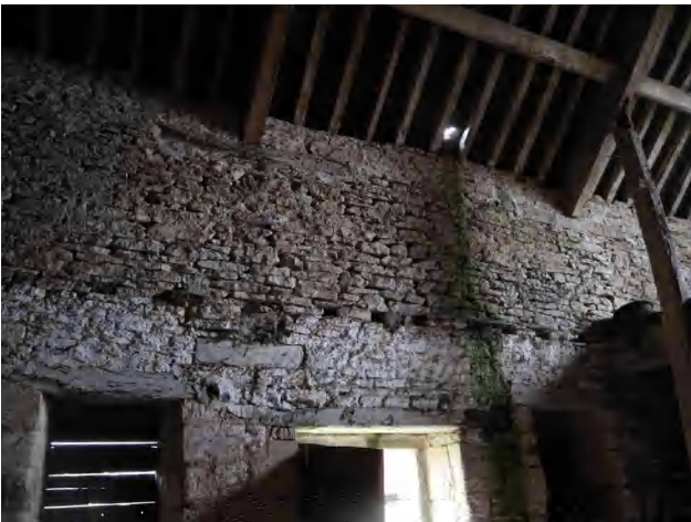
3.31 Building B, south wall, showing empty sockets in the wall, and timber bearer for now-removed transverse beam (DIA).
