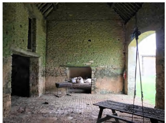
3.13 Building A, east end. General view looking west, showing brick floor section (DIA).
