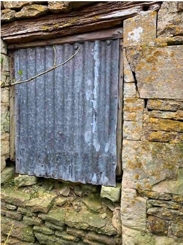
3.42 Window within former larger opening in the southern elevation of Building C (DIA).
