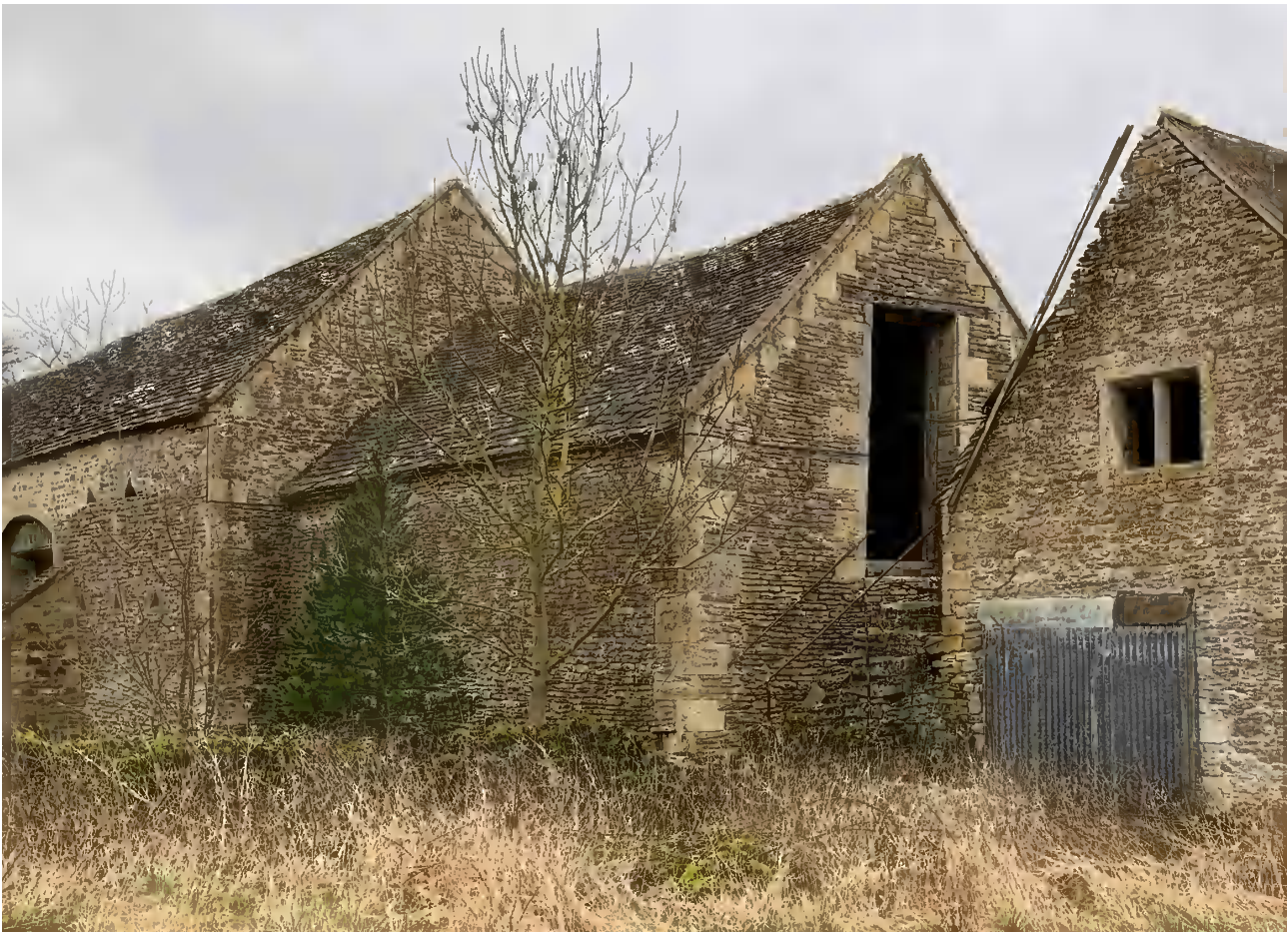
3.23 Building B from the north west, showing the north and west elevations (DIA).
