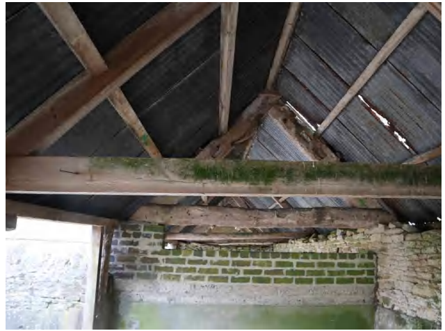
3.61 Building D, looking south, showing the northern dividing wall, and modern roof structure (DIA).
