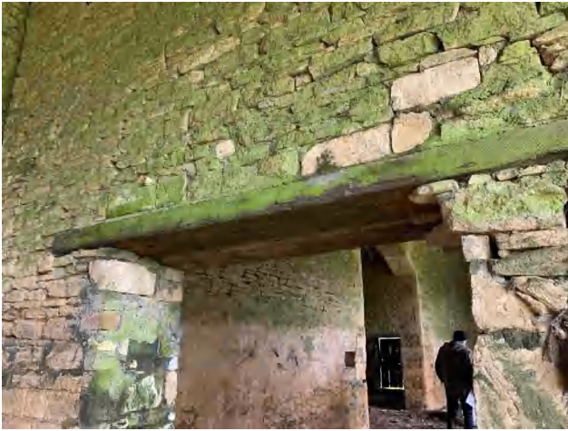
3.16 Building A, east end, detail of 20 th century opening in the wall between the two parts of the building (DIA).
