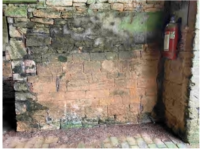
3.15 Ashlar wall construction to the north of the opening between the two parts of Building A (DIA).
