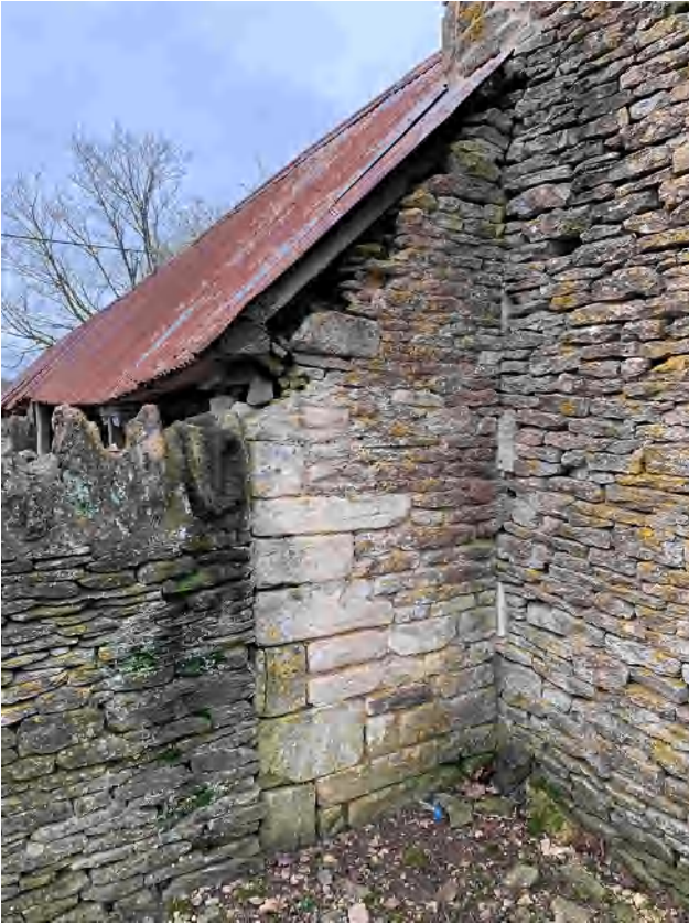
3.57 Part of the northern end wall of Building D, showing its junction with Building D, and with the drystone enclosure wall (to the left) (DIA).
