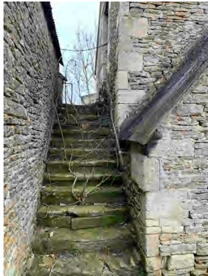
3.25 The southern tallet steps, from the south - building B is on the right, Building C on the left (DIA).
