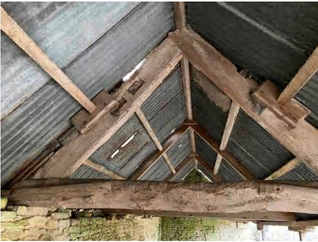
3.59 The roof of the northern part of Building D, from the central part (DIA).
