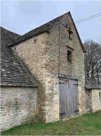
3.5a Building A - eastern porch and pigeon loft from the south west (DIA).
