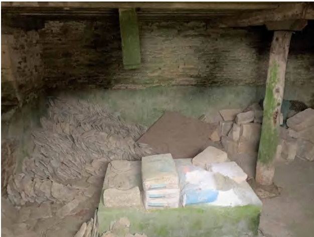
3.51 View into the ground floor of Building C from the gap above the door in the east elevation. The chute is in the centre, and the reveal of the window in the south elevation is on the left (DIA).
