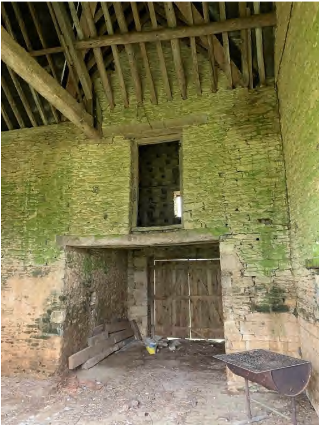
3.18 Building A, east end. Entrance to porch, with pigeon loft above (DIA).
