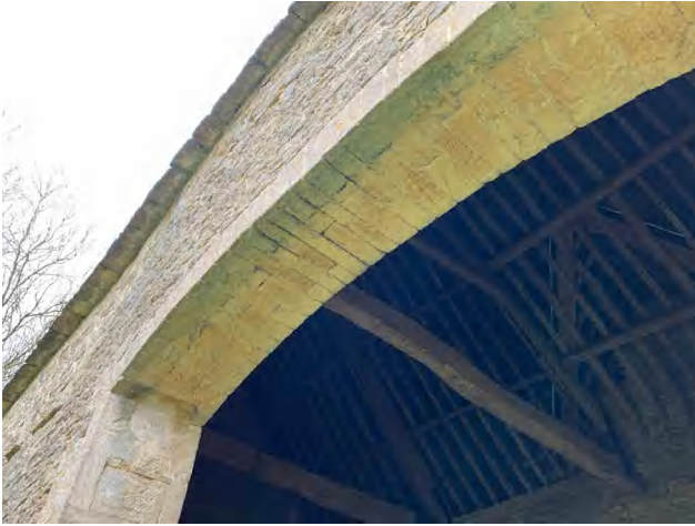
3.14 Building A, eastern end, soffit of northern entrance arch, and roof structure within (DIA).
