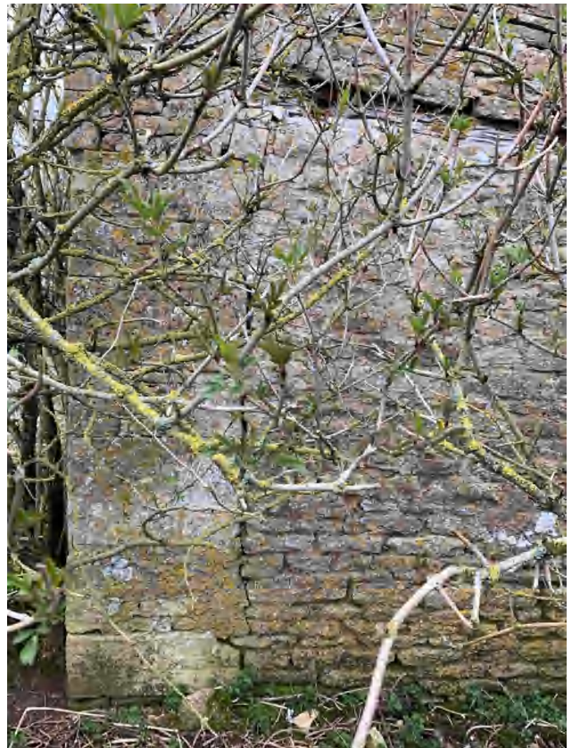
3.43 Straight joint and lintel showing the former extent of the doorway (left side) in the south elevation of Building C (DIA).
