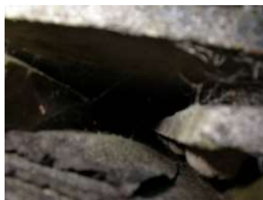
Fig. 14 Holes cobwebbed and dusty
