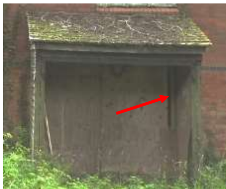
Fig. 35 Gap to the side of the lower entrance door
