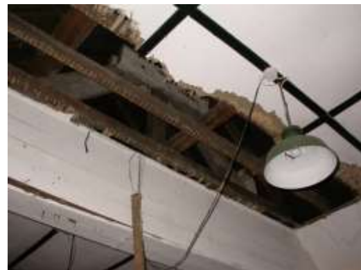
Fig. 18 Hole in ceiling of western room
