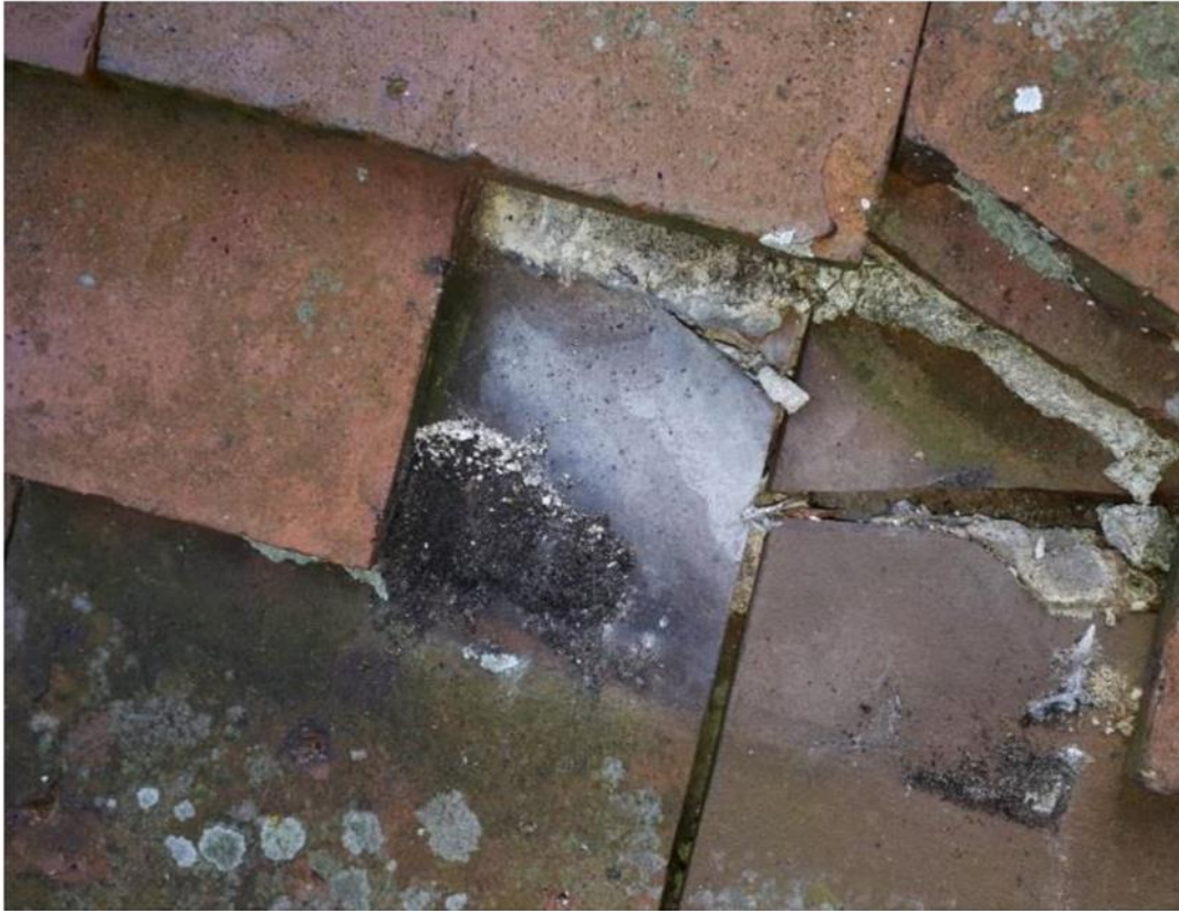
Lichen growth on roof tiles and severe frost damage
