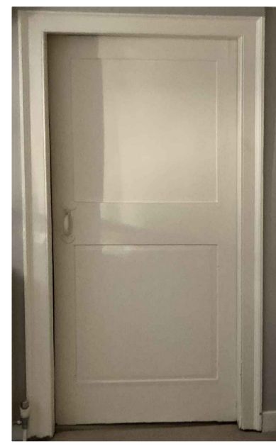
Existing second floor landing door to be retained and made good. New door to match the existing
