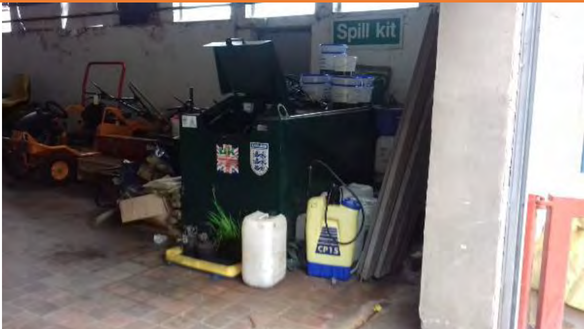
PLATE 2: DIESEL STORAGE TANK
