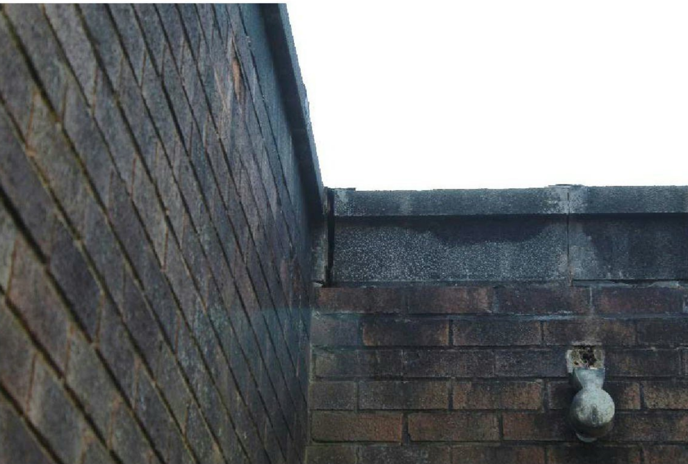
Gap between the coping stones - filled with dense cobwebs
