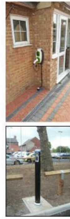
Electric Vehicle Charging Station Refer to Site Plan for locations of charging points.
