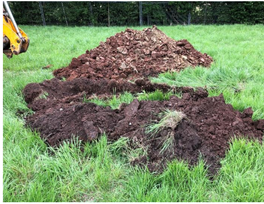
Photograph 1 – Displaying arisings at SA01, Topsoil and Made Ground (near side) along with the underlying Mercia Mudstone Group (far side).
