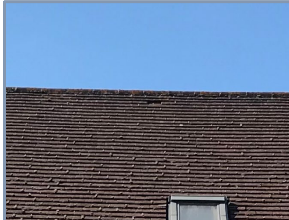
Photograph 2: Missing tile on the eastern aspect of B1
