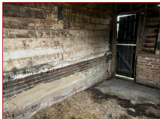
Photo 18: View within northern annex looking at North elevation of principal barn
