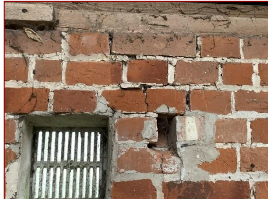
Photo 26: Cracking in Masonry to East Wing
