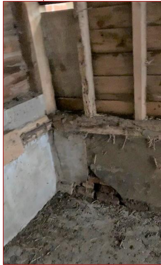
Photo 34: Separation of eastern plinth from southern plinth to main barn
