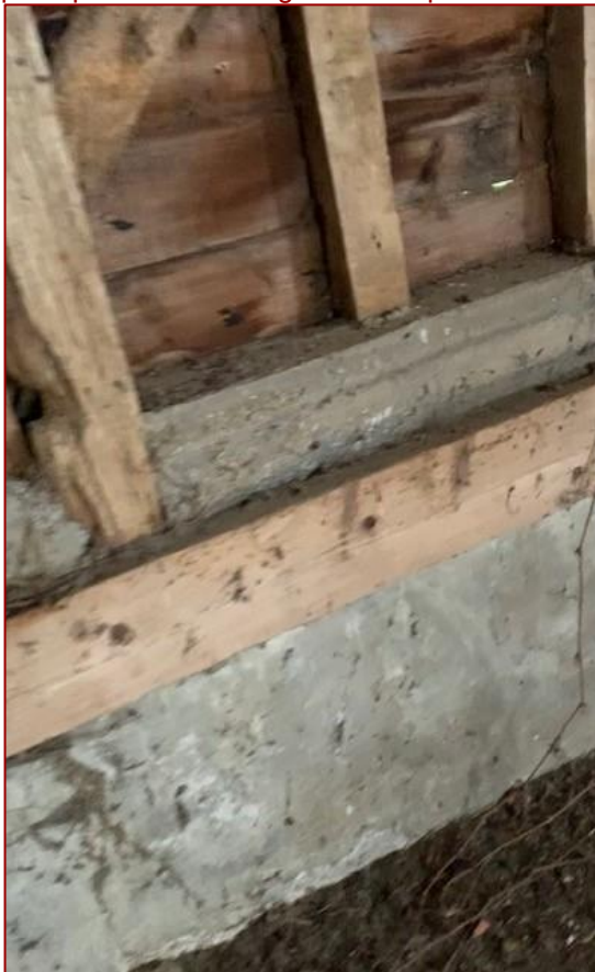
Photo 33: View of rendered plinth and concrete encasement to wall plate on east elevation
