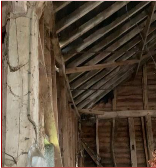
Photo 31: View along north elevation along principal barn showing lateral displacement
