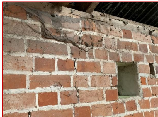
Photo 24: Cracking in Masonry to East Wing
