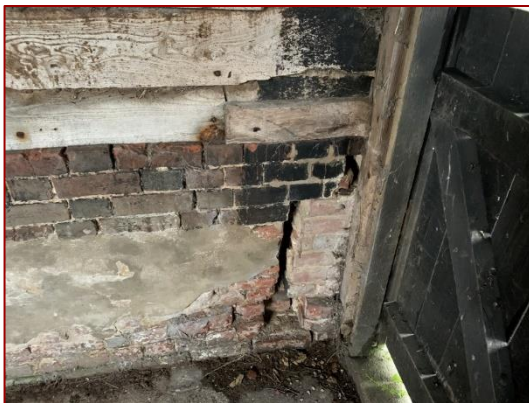
Photo 27: Separation of Western Gable Plinth from Northern Plinth to principal barn
