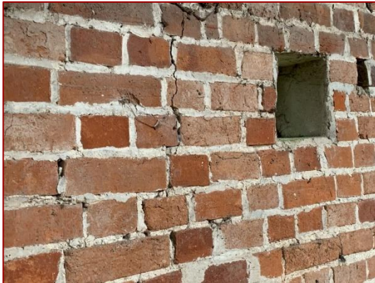
Photo 25: Cracking in masonry to East Wing
