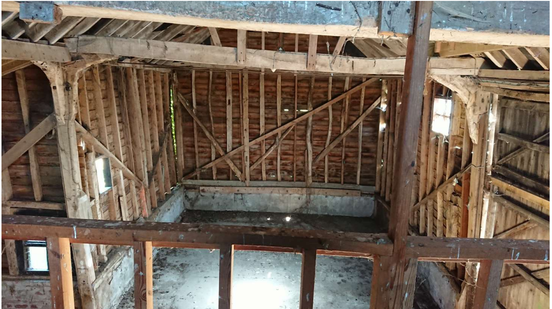
Internal frame view
