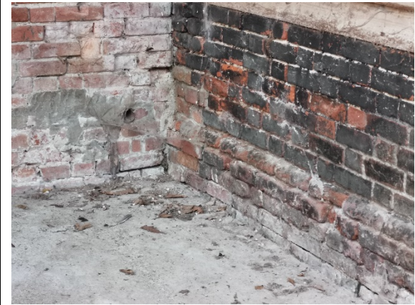
Damaged brickwork in the stables
