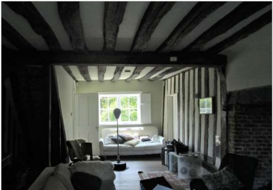
Fig. 5: Early C15 parlour wing looking east, with original medieval stair to left and later fireplace to right. The door in the studwork wall beyond leads through to the lean-to structure which is the subject of this application.
