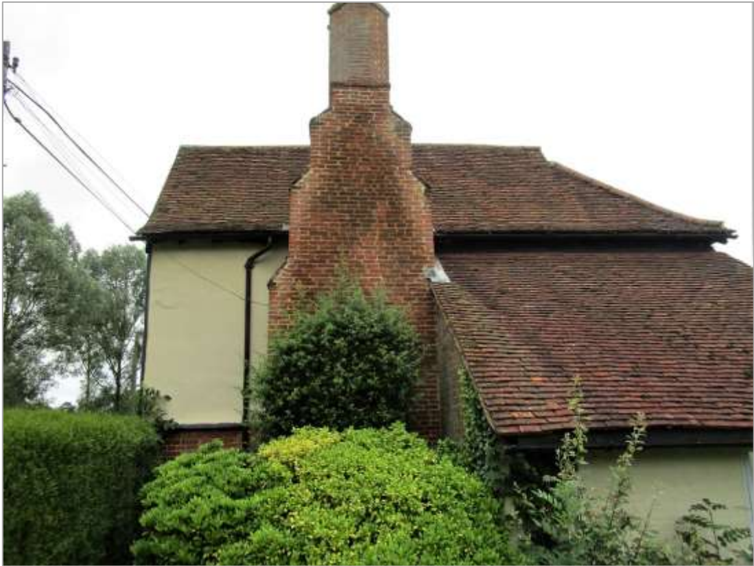
Fig. 4: Brick stack added to the parlour range in the C16. The upper part of the stack was rebuilt c.2000. Alongside the stack is the C20 lean-to addition to be removed under current proposals.
