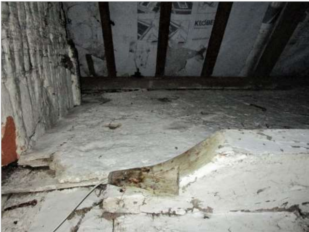
Fig. 15: View upwards through a small trapdoor in the ceiling into the roof space of the lean-to. The timber in the foreground is of uncertain purpose but may represent a wall plate belonging to a previous roof. Below this (still within the roof space) the studwork of the originally outer wall of the parlour range is exposed and limewashed. Above it, old plaster is still present over the C15 timber framing. To the left is the side of the C16 brick stack, and above is the modern roof with sawn timber rafters and roofing felt.
