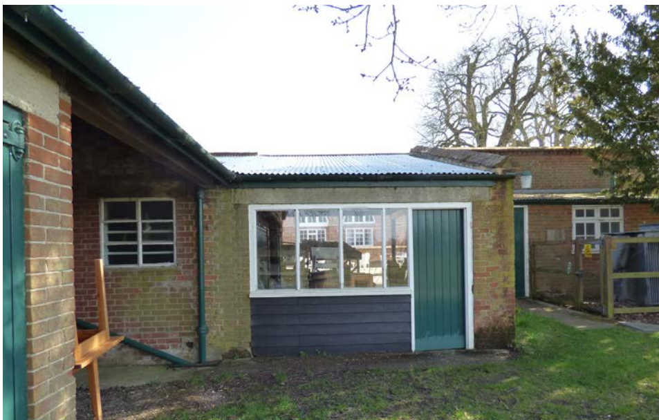
Potential infill to be removed, to allow a more direct connection between stable yard, park and potential shop. Note existing substation and gents WCs to right
