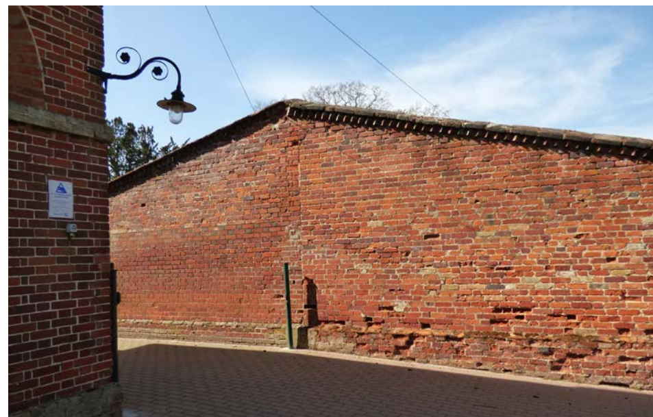
Southern end of North-East Stable range: Note multiple phases of brickwork apparent
