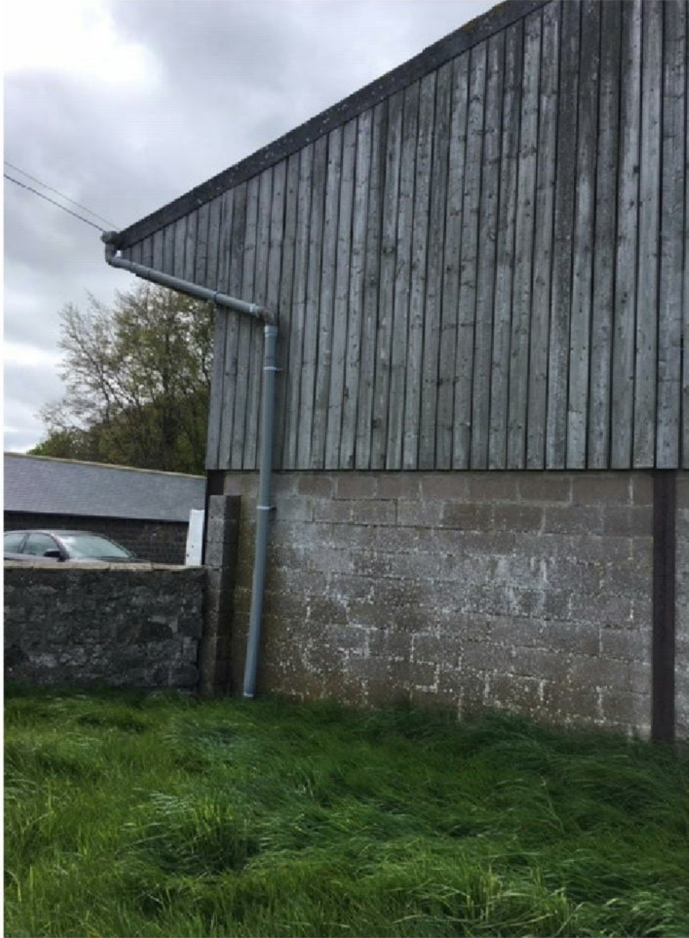
Photograph Showing RWP in South East Corner Discharging into Sewer
