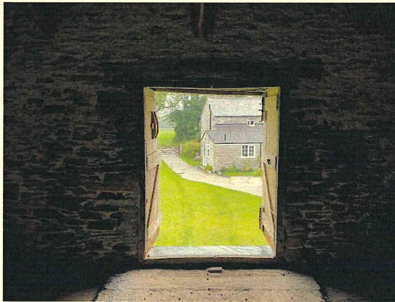
Photograph 18 – View on front hay loft door opening at first floor level with timber lintel over.
