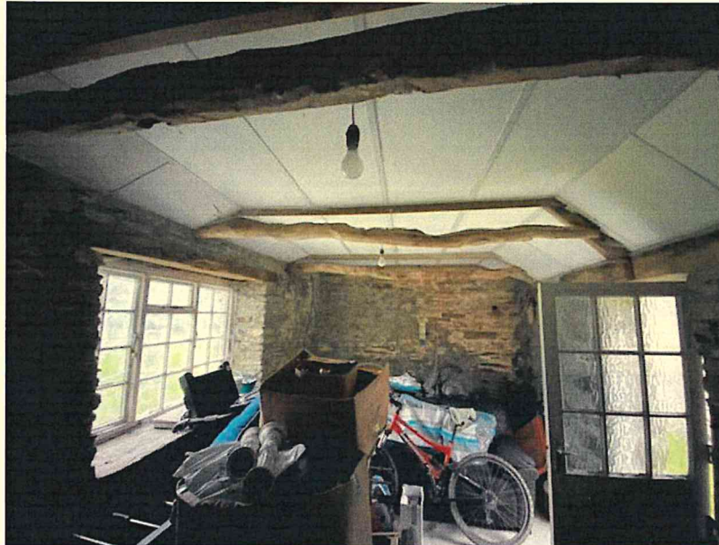
Photograph 29 – Internal view on ceiling boarded roof structure to west end of barn.
