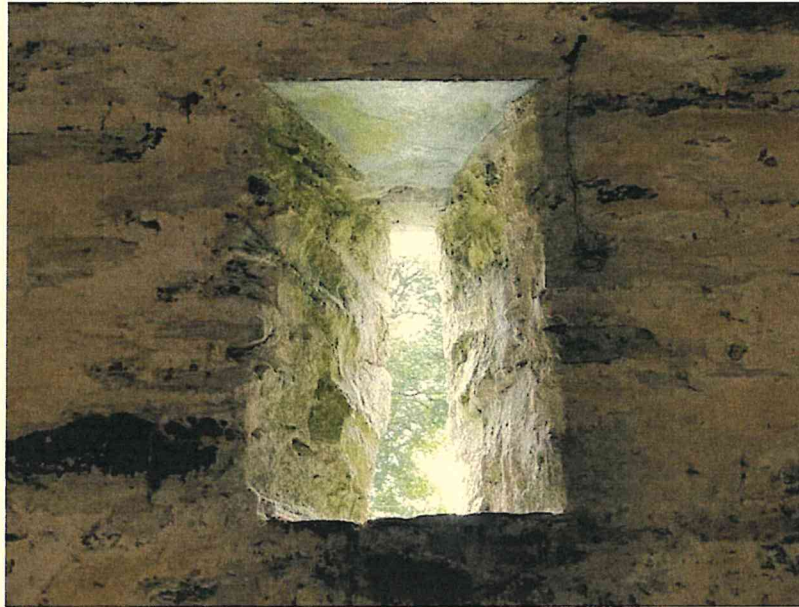
Photograph 20 – Arrow slit window opening at high level on gable with stone lintel over.
