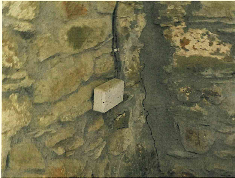
Photograph 25 – Internal cracking at flank to gable wall return, filled with cement, reopening.
