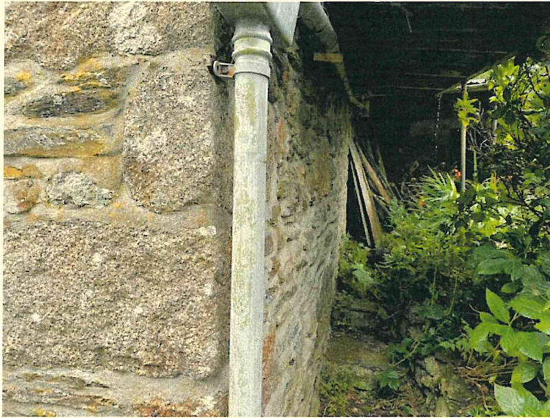
Photograph 2 – Isolated lateral movement of stonework at rear corner.
