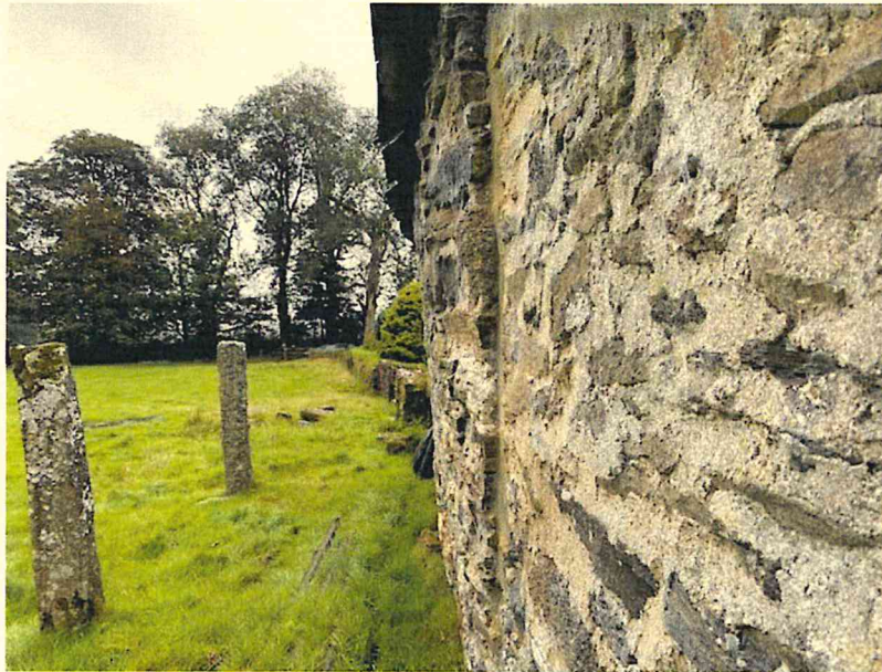
Photograph 23 – Extent of outward displacement on western end rear flank wall.
