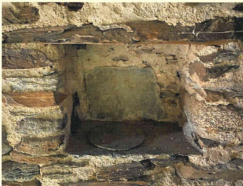
Photograph 19 – Alcove to right side of door opening with stone lintel locally over.
