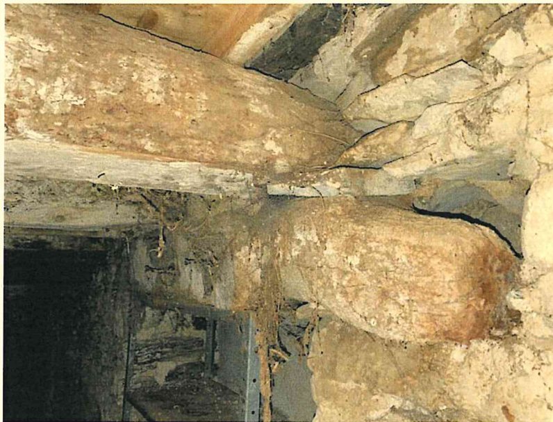
Photograph 17 – Displacement of lintel over rear ground floor door opening.
