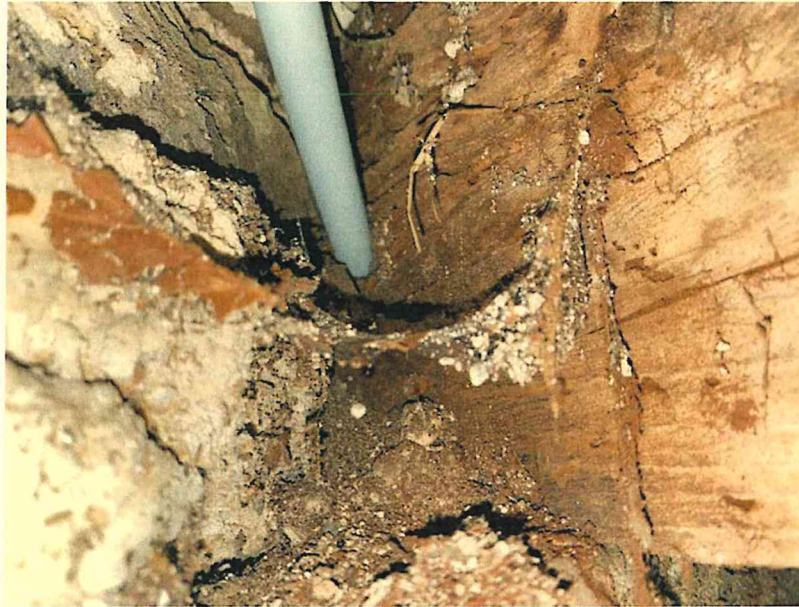
Photograph 8 – Rotten joist end at bearing on rear wall.
