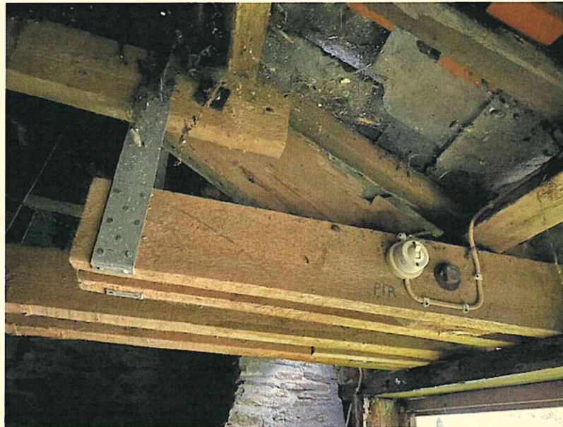
Photograph 28 – Ad hoc timber and bracket repairs to truss bearing on front elevation.
