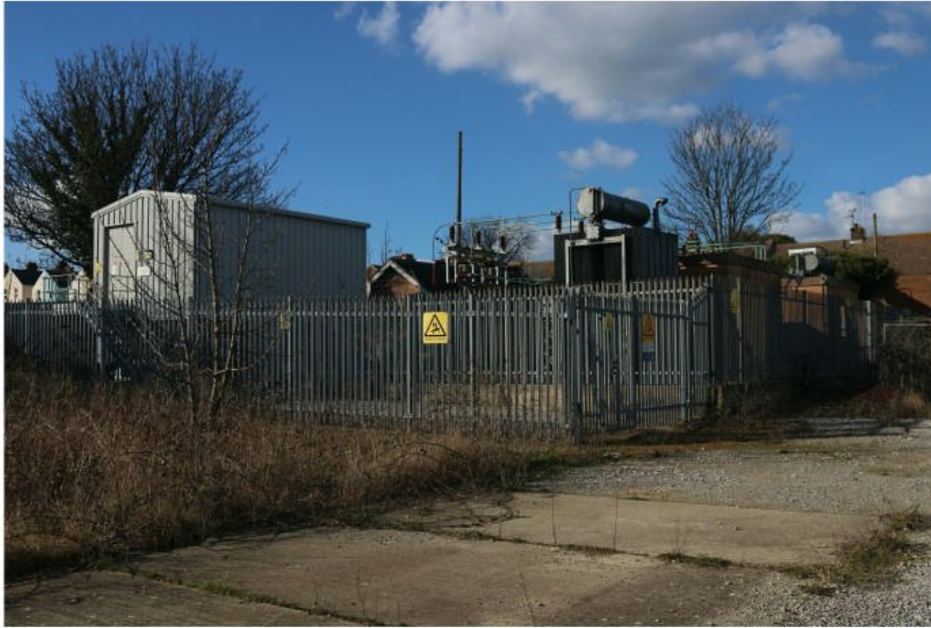
Electricity Sub Station on Western Boundary
