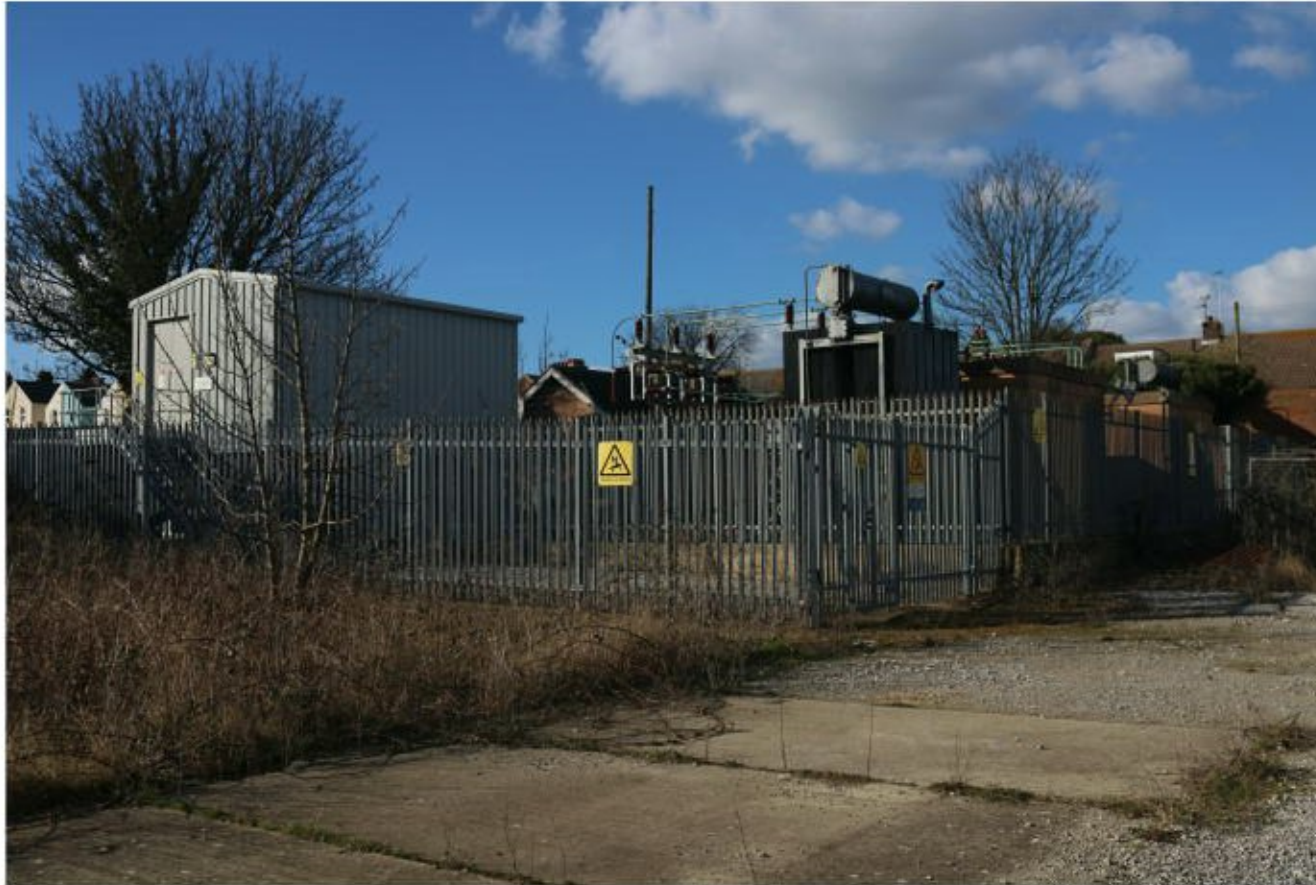
Electricity Sub Station on Western Boundary
