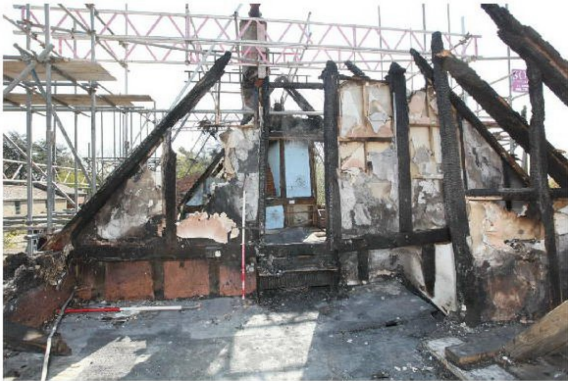
Illus. 25. The chamber above the probable parlour from its gable to the north-west showing the fully framed partition adjoining the central hall chamber. The jamb of the original ground-floor door lies close to the storey post on the left with a pegged short stud above the lintel and the first-floor door is an insertion between to original studs. The floorboards consist of recent softwood throughout the upper storey with no evidence of earlier boards beneath.
