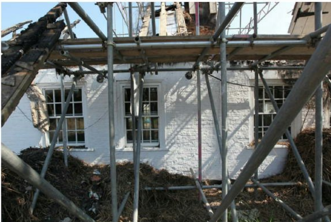
Illus. 2. A detail of the south-western facade showing its painted Flemish Bond 19 th century brickwork and sash windows. The closers (quarter bricks) respecting the central window in this image continue to the ground alongside a vertical joint in the bonding, suggesting it occupies the position of an entrance that opened into the corner of the central door – corresponding to the path on the historic Ordnance Surveys and possibly indicating the location of the original entrance.
