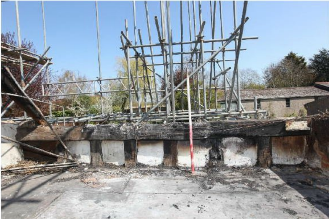
Illus. 35. The exposed original framing of the rear, north-eastern wall of the probable service chamber, immediately above the ground-floor window shown in illustration 19. The chamber would have been lit by a window in its missing gable matching that of the north-western chamber. A dovetail joint for a missing tie-beam that defined a narrow bay for the original chimney is visible on the left (illustration 36).
