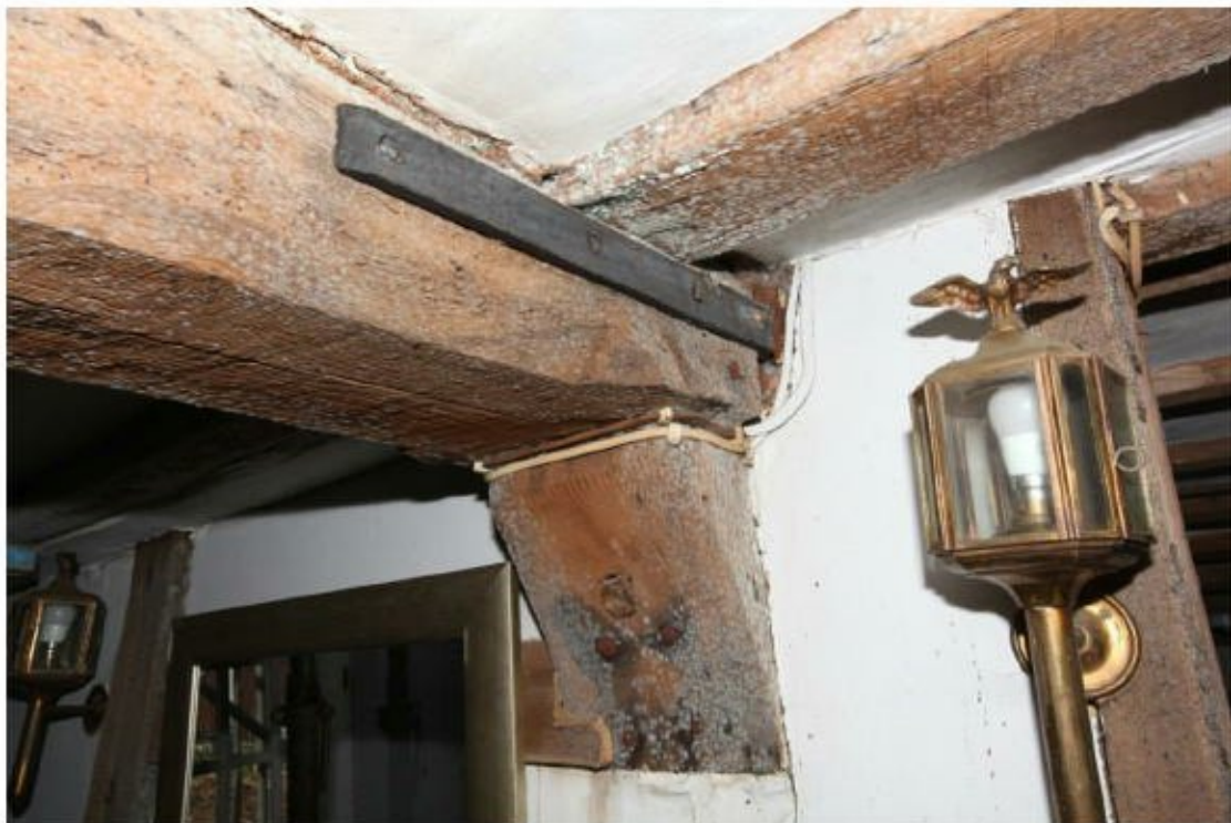
Illus. 8. A detail of the neatly curved chamfer stop to the south-eastern end of the hall's axial joist in the style of the late-16 th and early-17 th centuries. The joist is supported by a shaped and chip-carved bracket attached to the rendered brickwork of the chimney.
