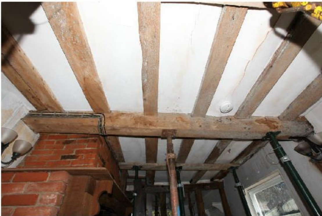
Illus. 16. The ostensibly original ceiling of the probable service bay showing its south-eastern gable on the right and the 19 th century chimney to the left. The chamfered and stopped axial joist respects the original chimney to the extreme left and appears to be tenoned to the remains of a central post in the gable on the right.
