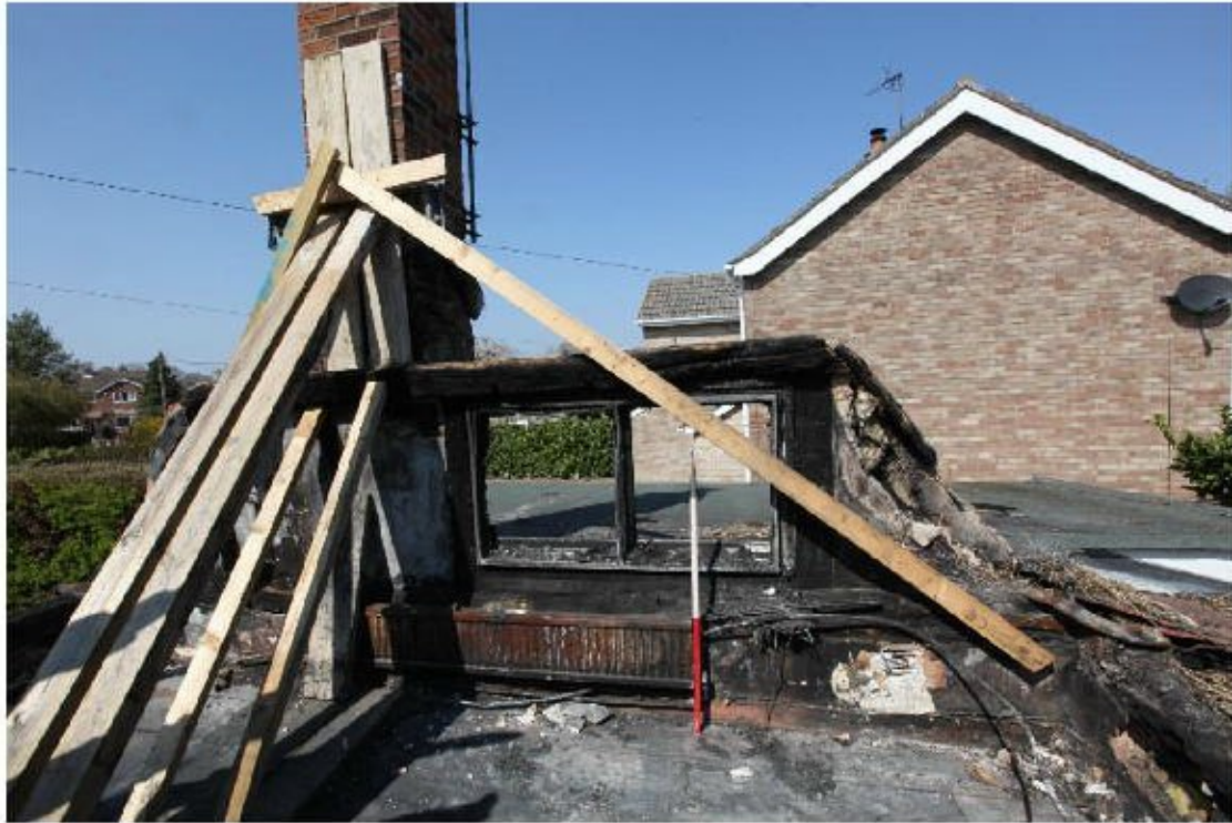
Illus. 23. The half-hipped north-western internal gable with evidence of an original window to the right of its centre in the underside of the upper tie-beam. The principal tie-beam is intact but largely hidden and any original studwork beneath is concealed by modern plasterboard. This gable is reconstructed in figure 16.
