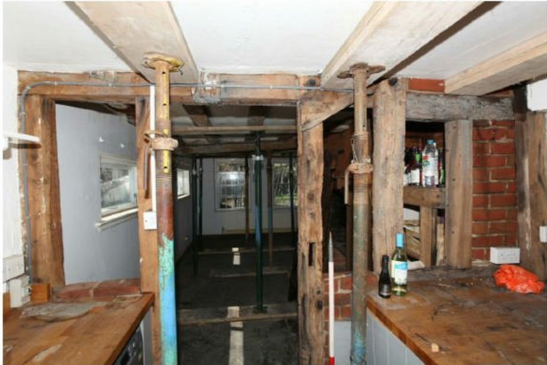
Illus. 21. The exterior of the parlour's rear wall from the lean-to kitchen extension showing two original truncated studs above the modern false studs on the left and a truncated original externally trenched wall brace against the central stud. The original window jamb and lintel are visible on the right.
