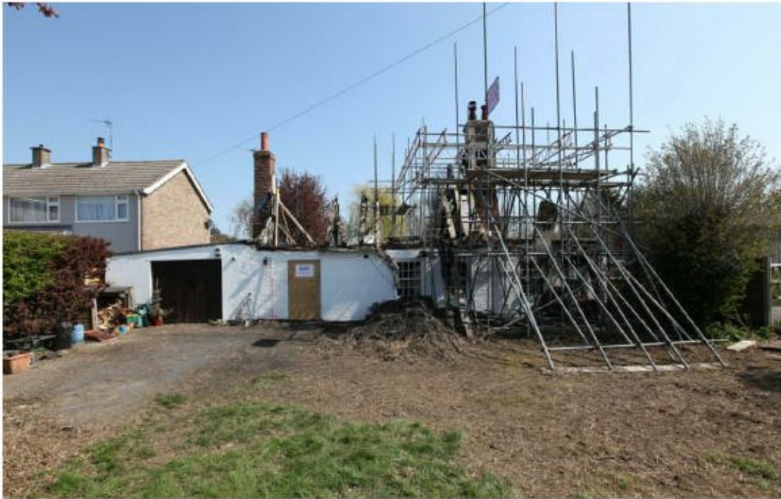
Illus. 1. The south-western facade with the 20 th century garage and the 19 th century chimney against the original north-western gable to the left.
