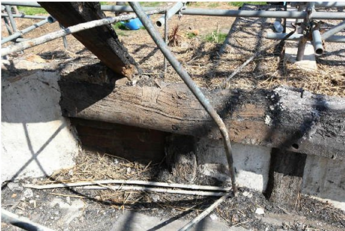
Illus. 36. A detail of the rear roof-plate in the south-eastern chamber showing a plaster-filled original dovetail joint for a missing tie-beam that formed a 1.1 m wide bay for the original chimney and corresponds with another in the front plate.
