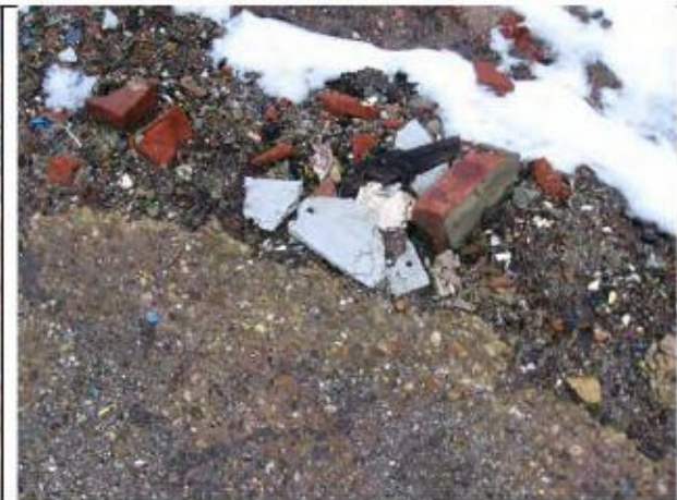
P3: ACM at ground level.
