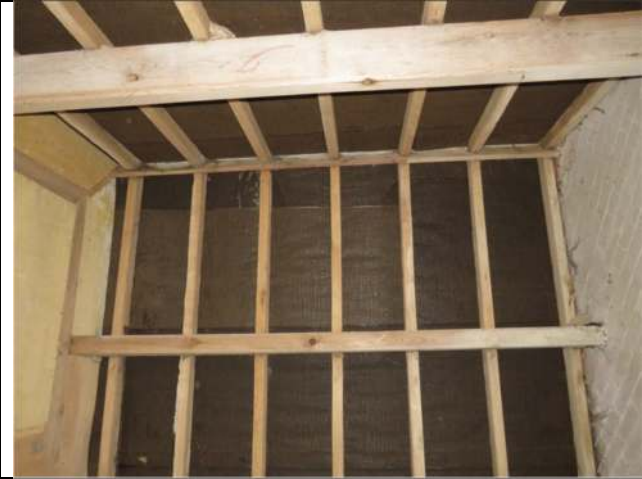
Photograph 13. The open roof void within the room to the north of the most southerly room within the Barn
