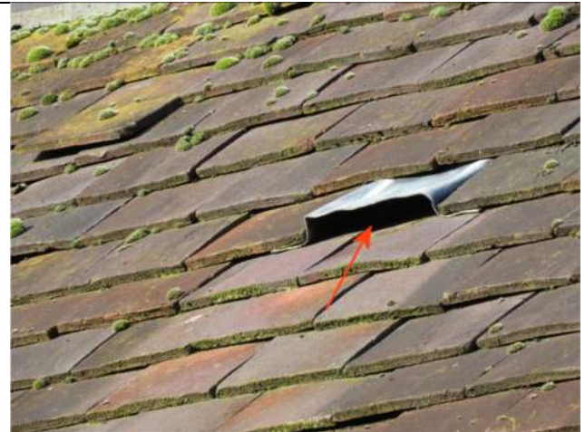
Photograph 4. Example of bespoke bat access into the bat loft within the Barn
