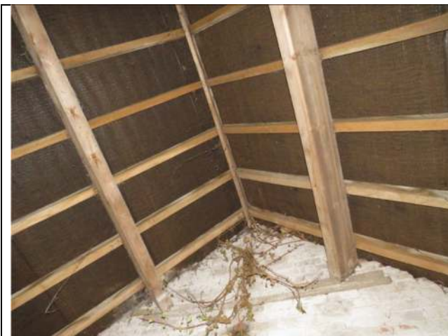
Photograph 11. The open roof void within the most southerly room within the Barn
