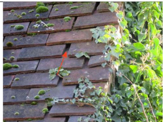
Photograph 6. Example of openings between tiles on the roof of the Barn
