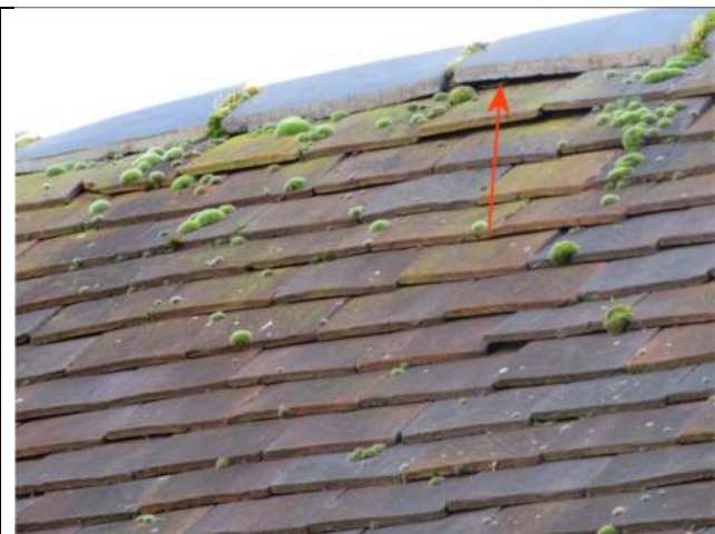
Photograph 5. Example of an opening under a ridge tile on the roof of the Barn
