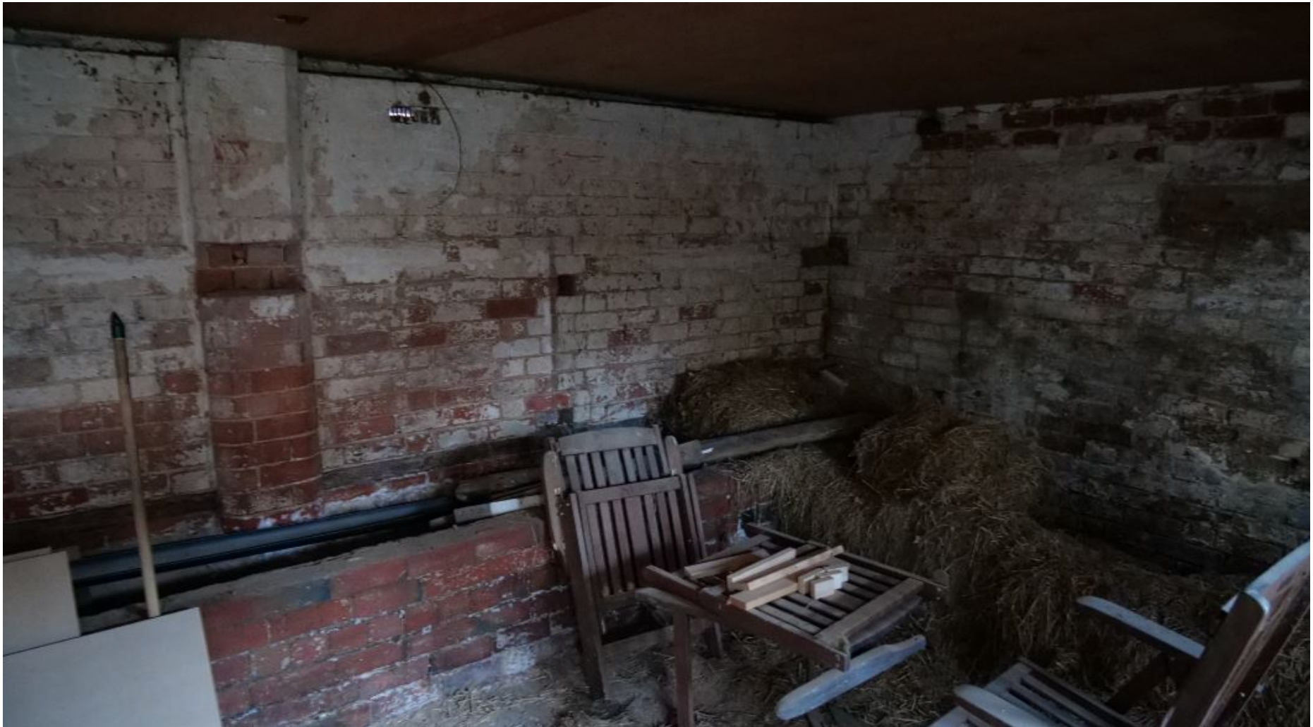
Figure 35: View of Feeding Trough – which originally ran along the whole of the eastern wall with the exception of the Cartshed Section of the Barn
