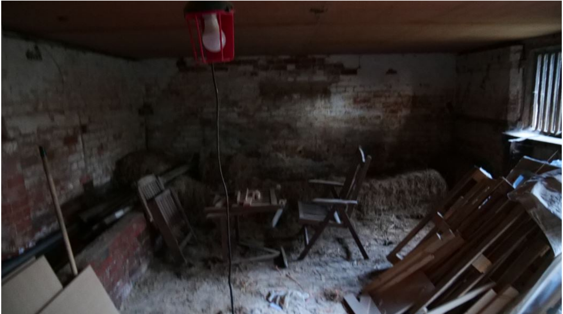
Figure 32: View of Northern End of Cowshed with Cattle Feeding Trough in Brick to left
