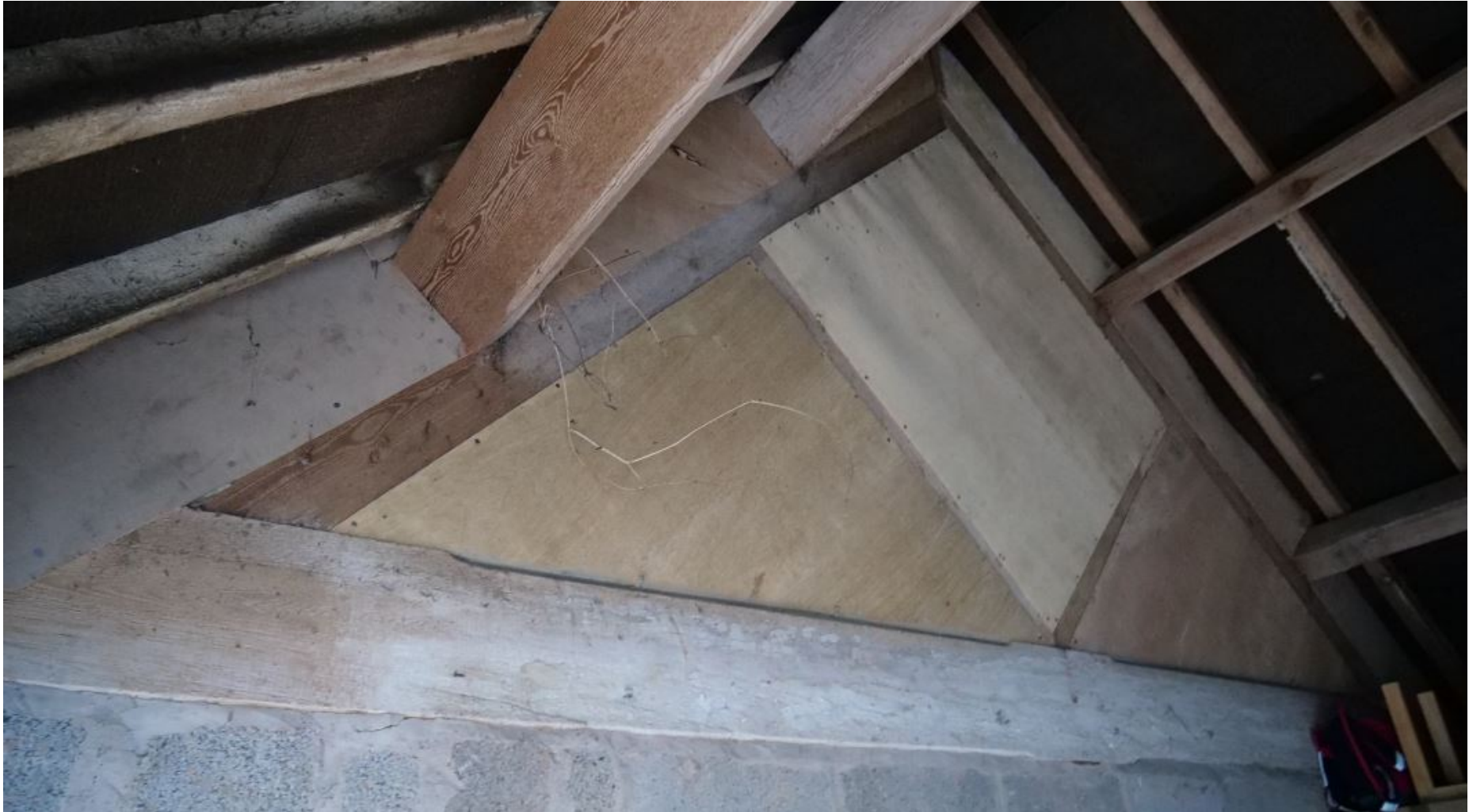
Figure 30: View of infilled timber truss (originally a King post Truss) above blockwork wall in C20 Garage
