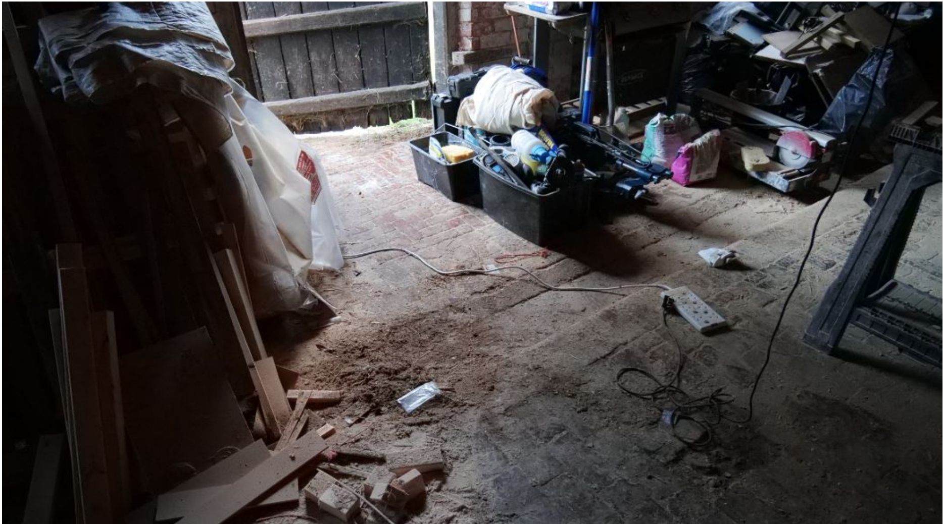
Figure 36: View of Floor of Cowshed
