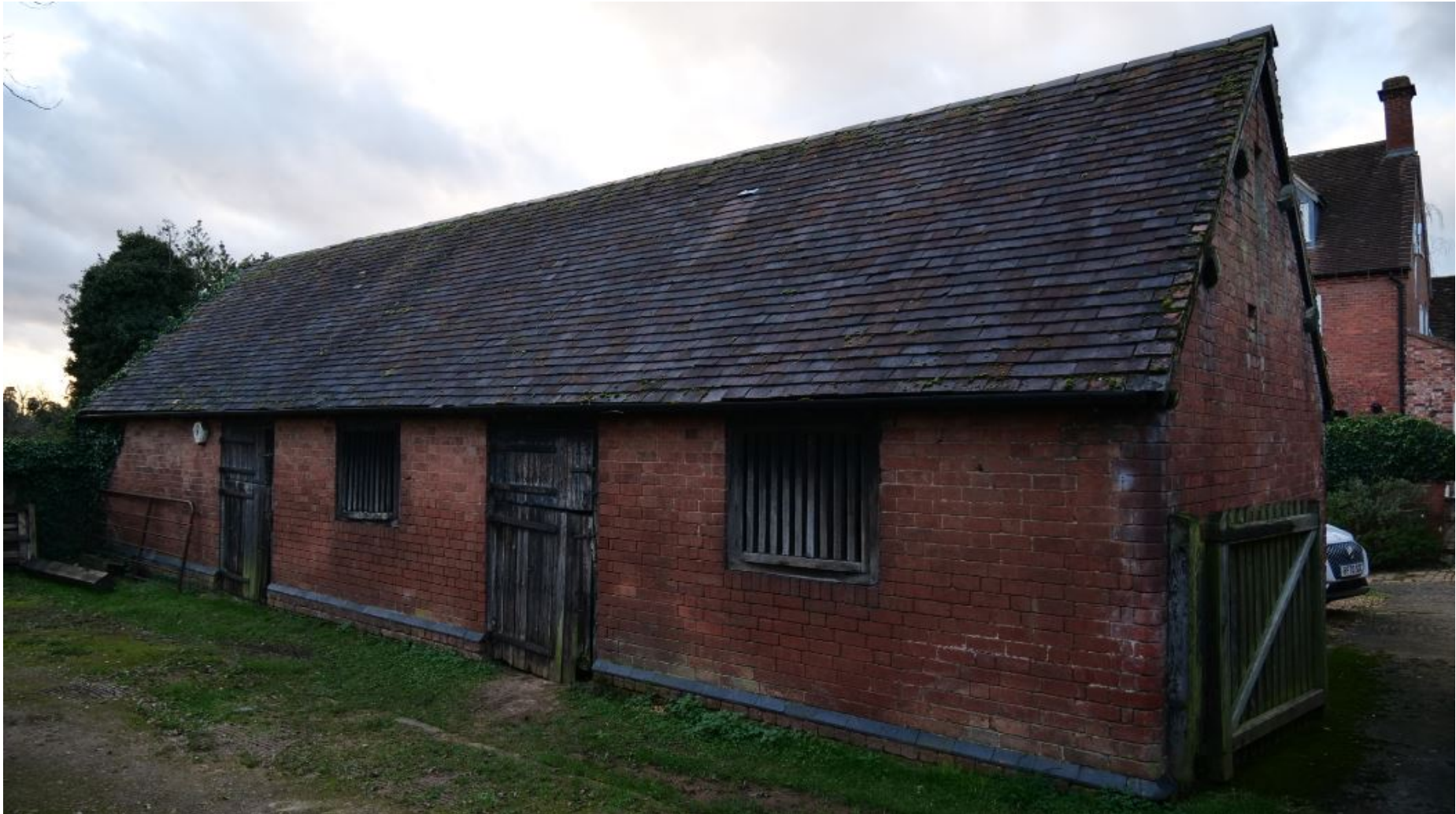
Figure 10: View of Barn Eastern Elevation with 2 original stable doors and 2 windows with timber grilles and no glazing
