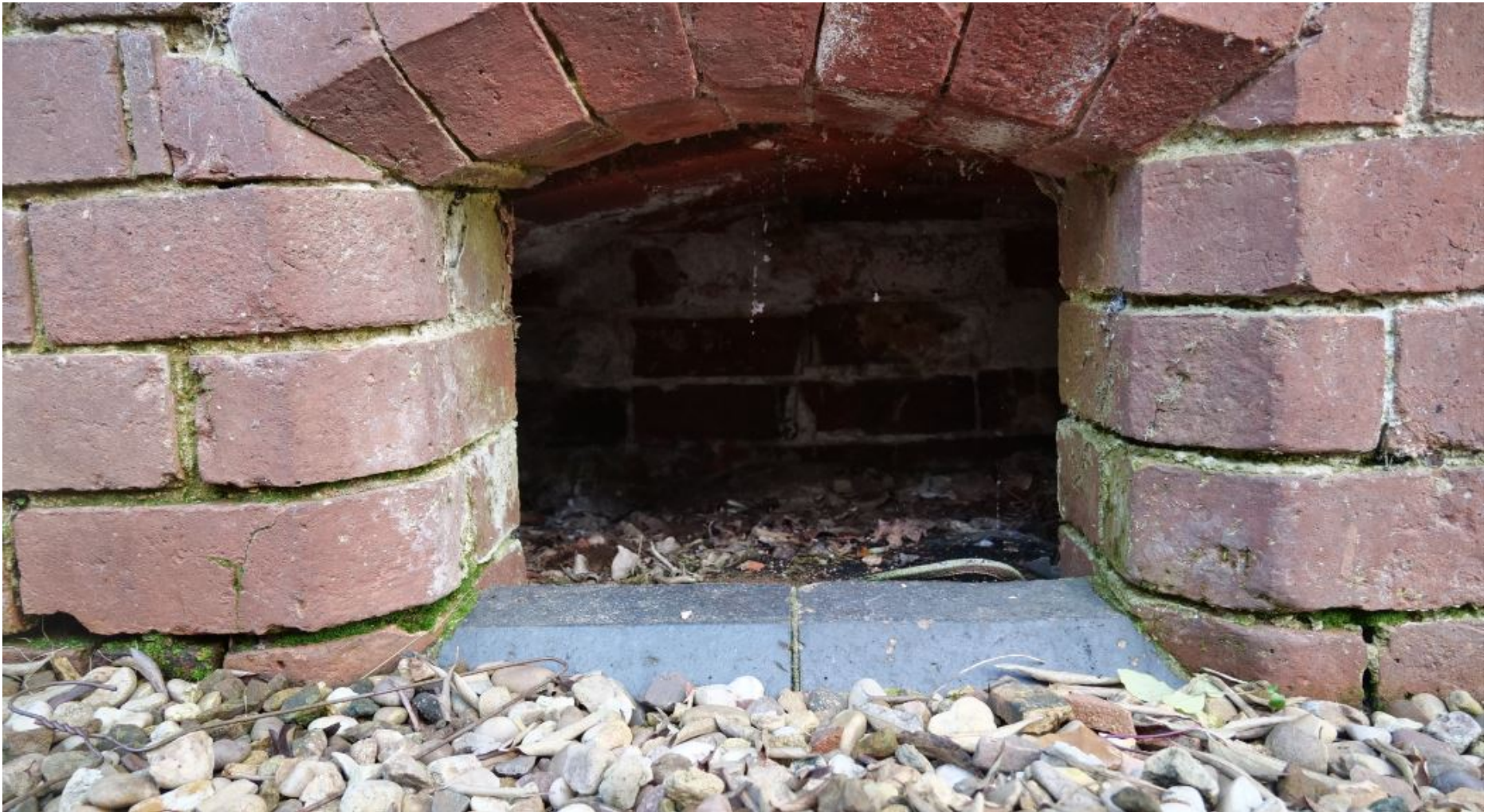
Figure 19: View of Hen Nesting Holes along base of Eastern Elevation of the Barn
