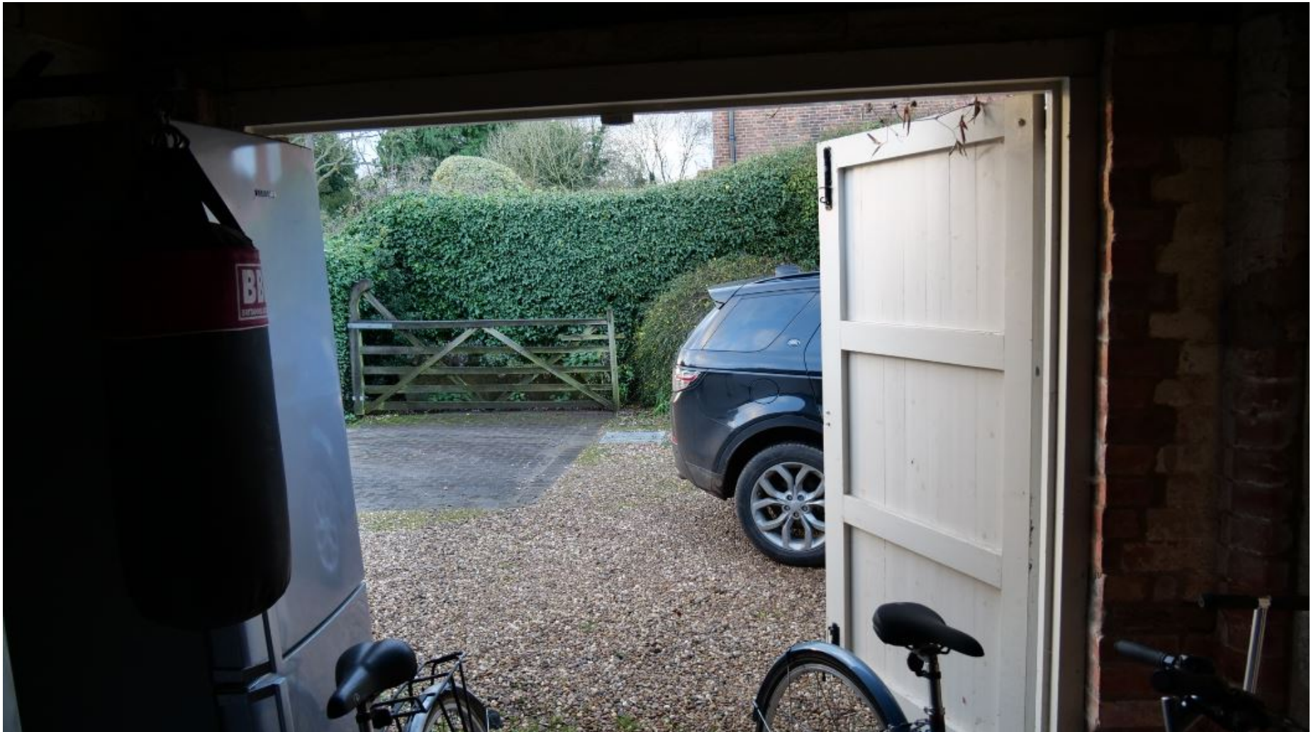
Figure 29: View of Out of C20 Garage with cut brickwork visible to the right of the doorway
