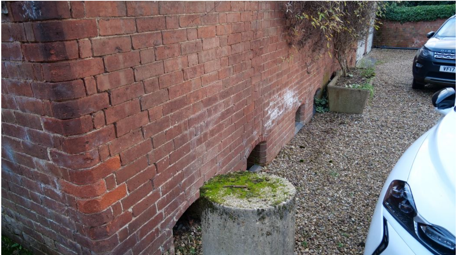
Figure 18: View of Hen Nesting Holes along base of Eastern Elevation of the Barn
