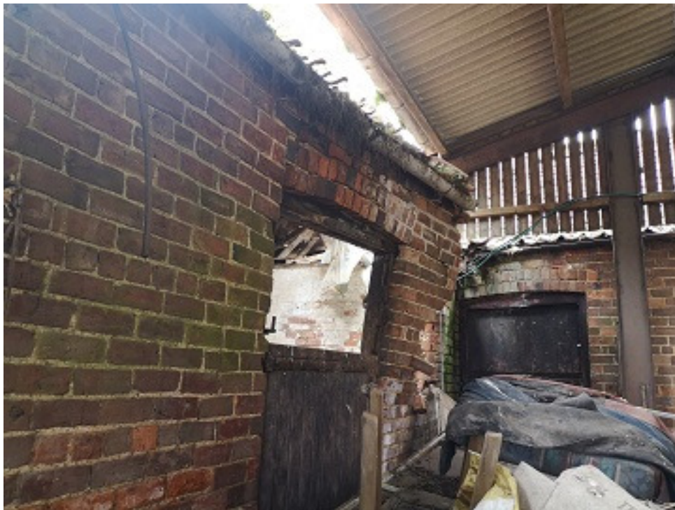
Plate 7. The eastern elevation of Building 5 viewed from within Building 8, with collapsing wall.
