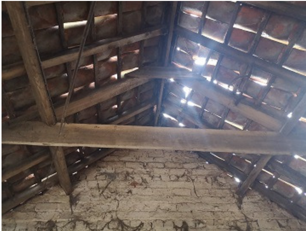
Plate 12. The timber roof structure and lifted/slipped tiles of building 7
