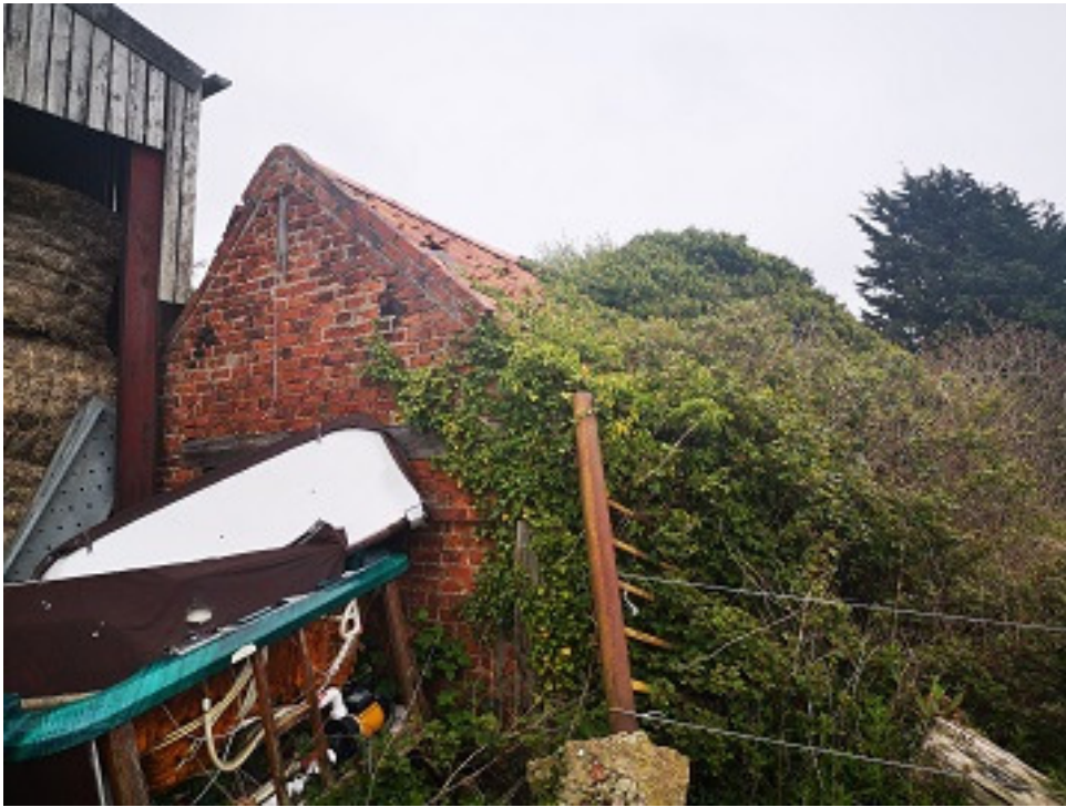
Plate 17. Common Ivy covering the east & south elevations as well as the majority of the roof.
