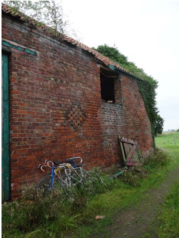
The above views are a selection taken along the western side of the main building which is currently all single storey.
