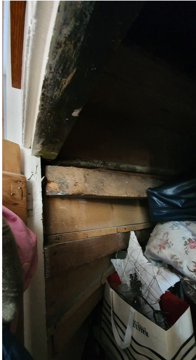
Photograph 7: Bearers and String attached to Newel Post (which forms the doorframe to the entrance to the staircase)
