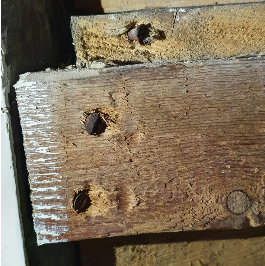
Photograph 10: Example of Different Fasteners in the Step Bearer
