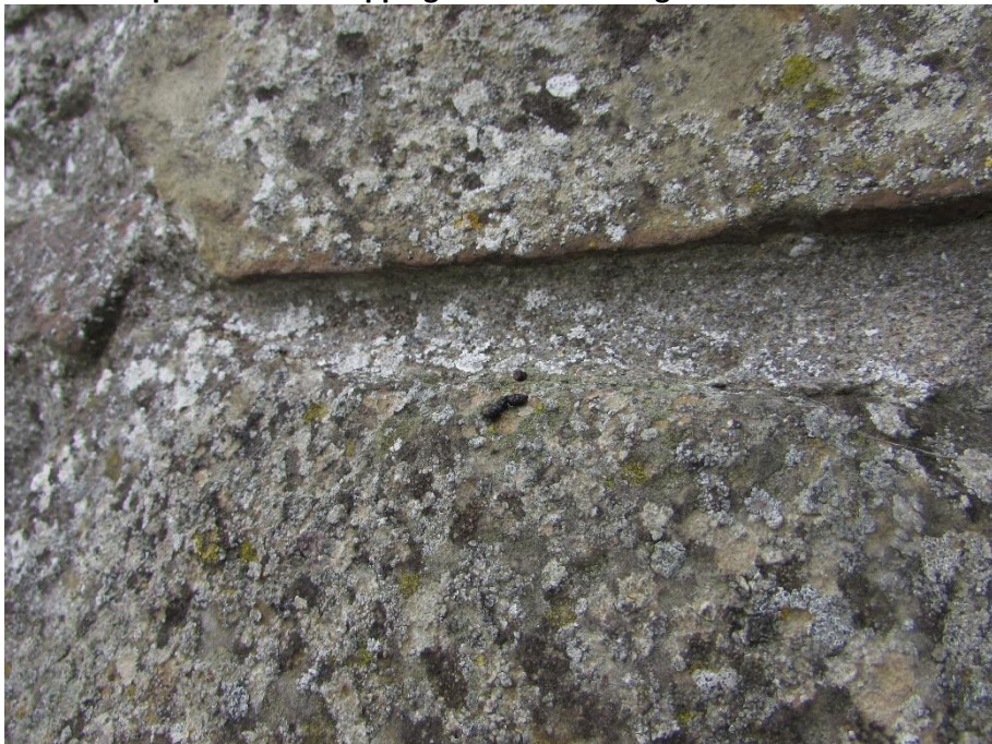
Plate 4 – Pipistrelle bat dropping found on north gable wall
