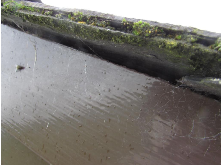
Plate 6 - Gap between the roof slates and the bargeboard of the north gable end
