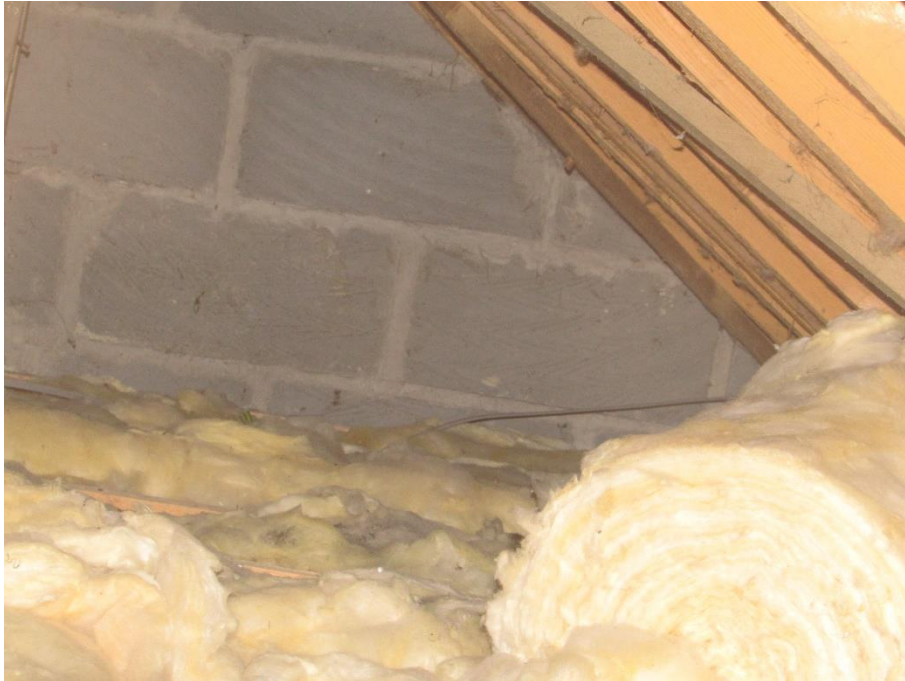
Plate 7 –Inside the north part of the loft – picture taken with zoom from the water tank
