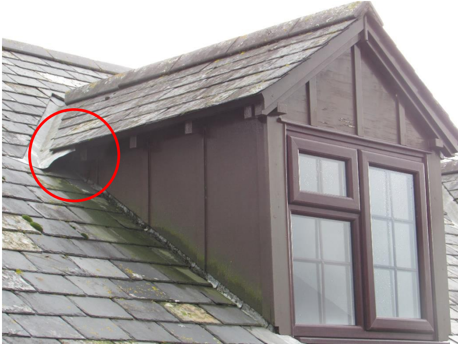
Plate 3 – Gap where the dormer intersects the roof
