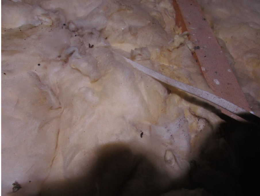
Plate 6 – Bat droppings inside the loft of the building
