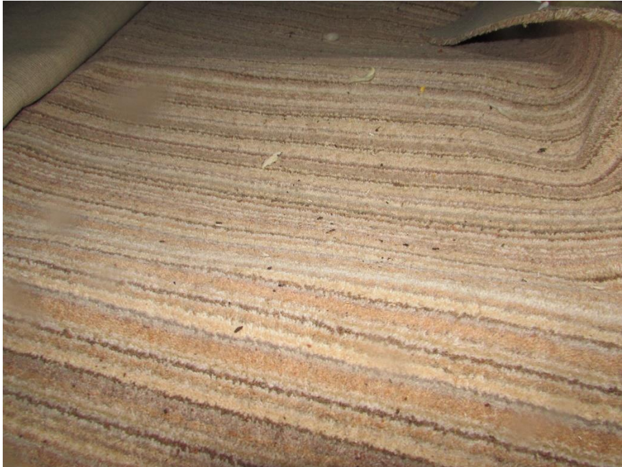
Plate 7 – Bat droppings inside the loft of the building
