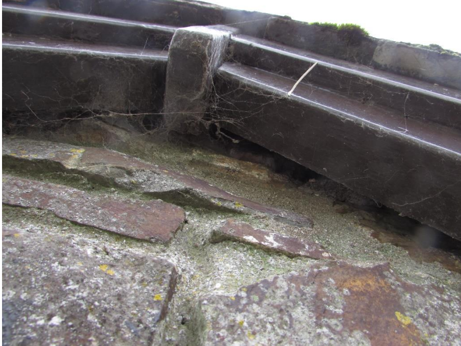
Plate 5 – Gaps above the north gable where the bat droppings found
