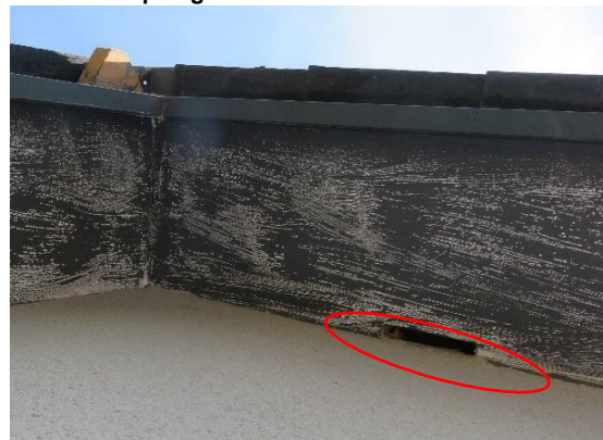
Plate 16: Gap at gable wall soffit
