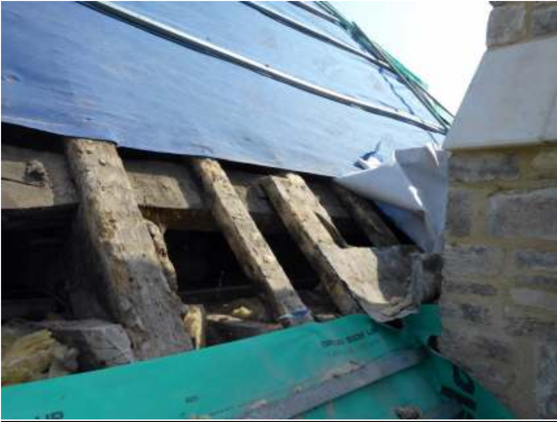
Original roof timbers visible. No alterations have been carried out to the roof timbers
