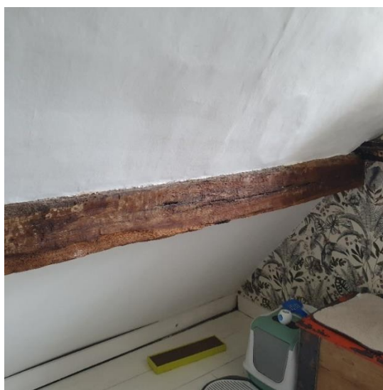
Beam in Bedroom 2
