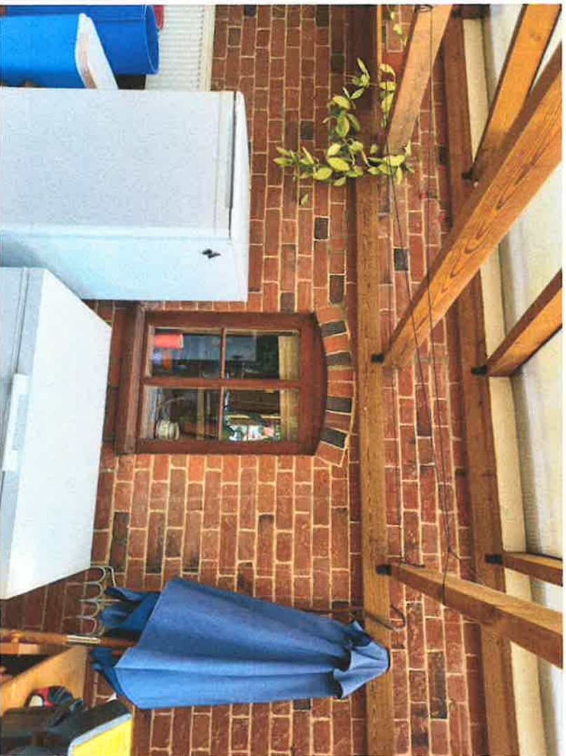
Rear wall of the main farmhouse within the extension – this wall will remain as exposed brickwork with holes repaired where roof timbers are removed.
