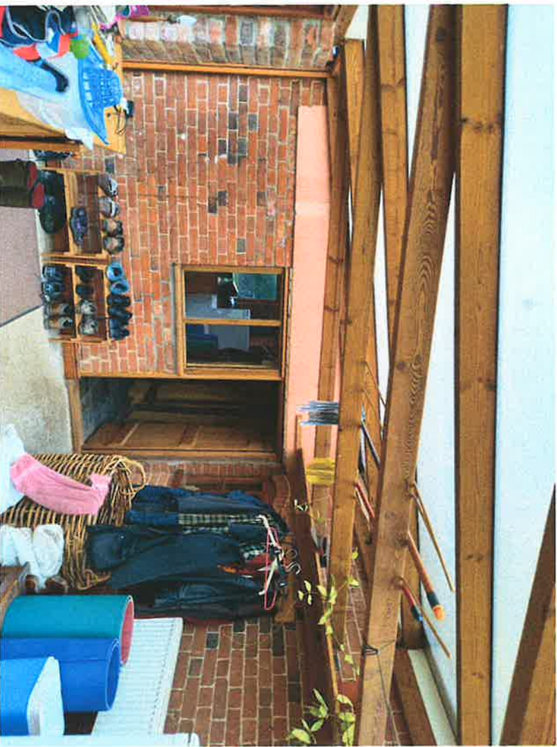
View of the inside of the existing structure – the pink render visible to the end wall will be removed and the whole of this wall plastered, together with the internal face of the new external walls to the extension.
