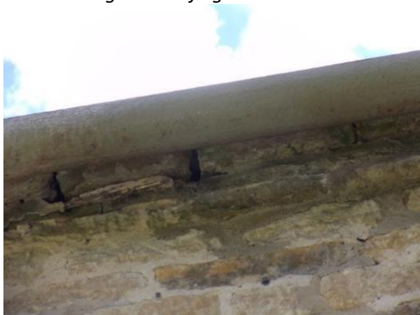
Plate 3.8: A few small gaps at eaves on western elevation
