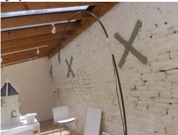
Plate 3.7: Interior of extension, sun room, with shallow gaps in stonework wall
