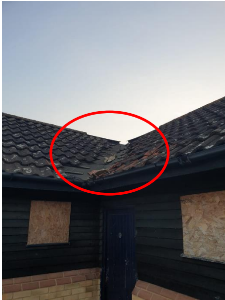
External tiles pulled off and smashed up on former loo block
