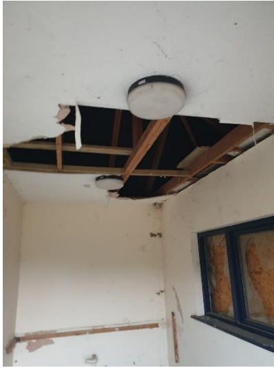
Internal vandalism in loo block (building 3)
