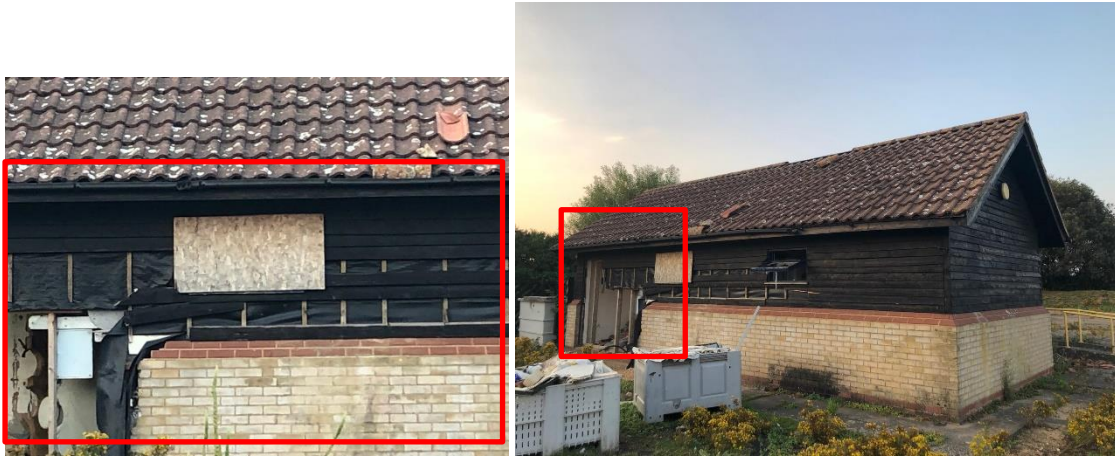
Panel boards pulled off, missing sections of walls
