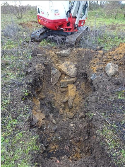
TP105 – Loose rubble made ground soils
