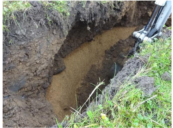
TP102 – Unstable loose sand beneath made ground
