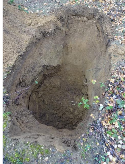
TP106 – Loose unstable excavation
