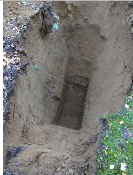
TP107 – Loose unstable excavation
