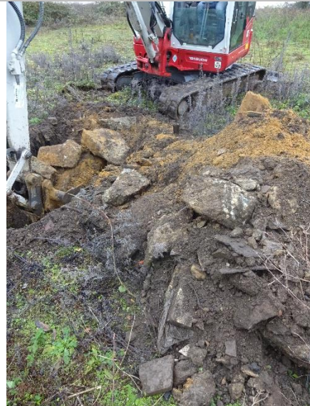
TP105 – Loose rubble made ground soils
