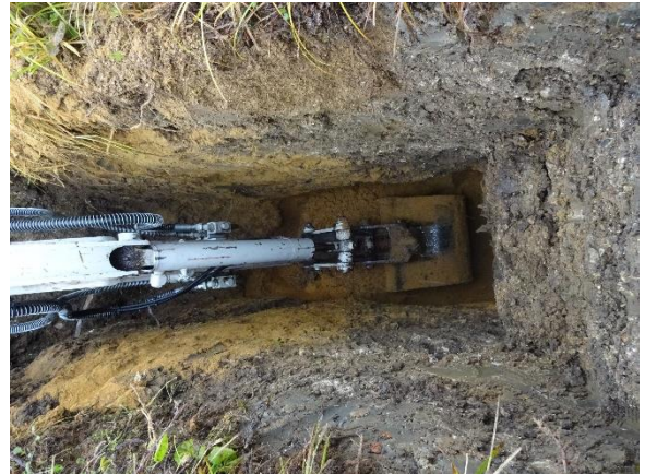
TP104 – Unstable loose sand beneath made ground
