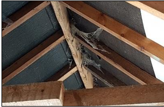
Figure 7: Roof lining and cobwebs throughout.
