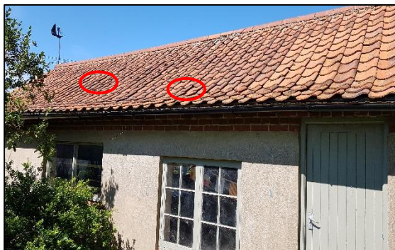
Figure 3: Gaps under tiles on southern aspect (circled).
