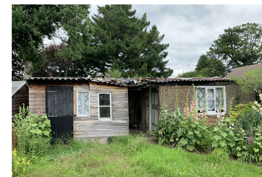
EXISTING GARDEN ROOM (DERELICT) - TO BE REPLACED.
