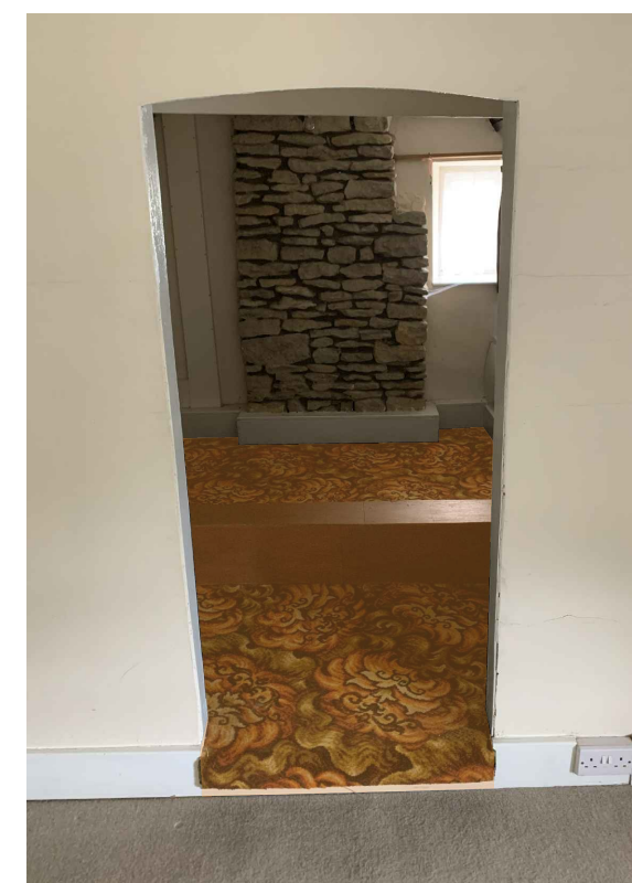
1970'S RAISED FLOOR TO ACCOMODATE SERVICES AND MODERN RAISED BOXING TO BE REMOVED.
